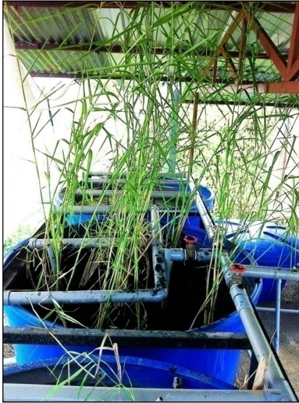
Figure 3.7 First stage of wetlands with two planted units (with Phragmites karka ) and one unplanted unit completed with pipe network for septage distribution (Wetland A1- A3)
