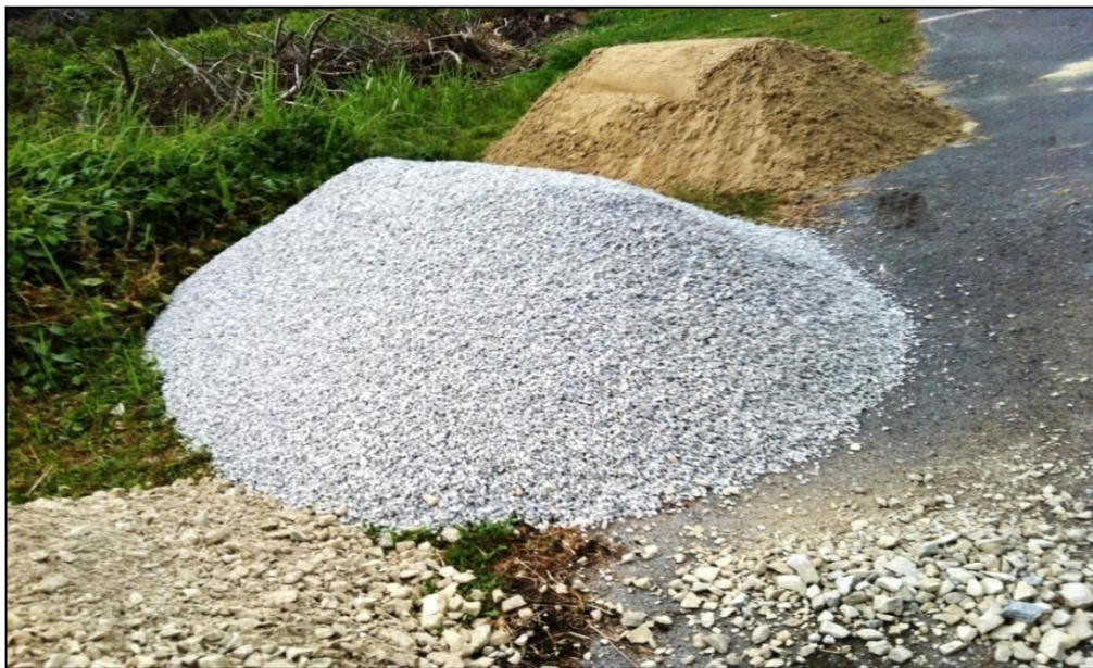
Figure 3.4 Sand and aggregates delivered to the project site for construction of wetlands
