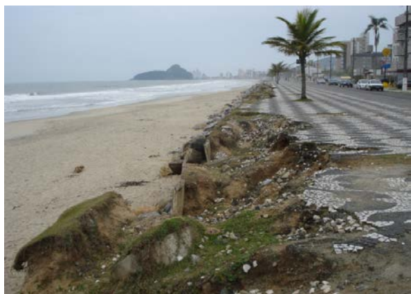
Figure 17: Sector V infrastructure problems.
