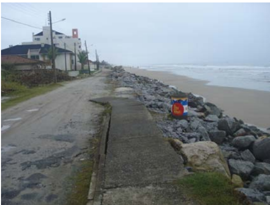
Figure 13: An example of how shoreline advancement causes damage to urban infrastructure, shown here by the damaged bicycle path.
