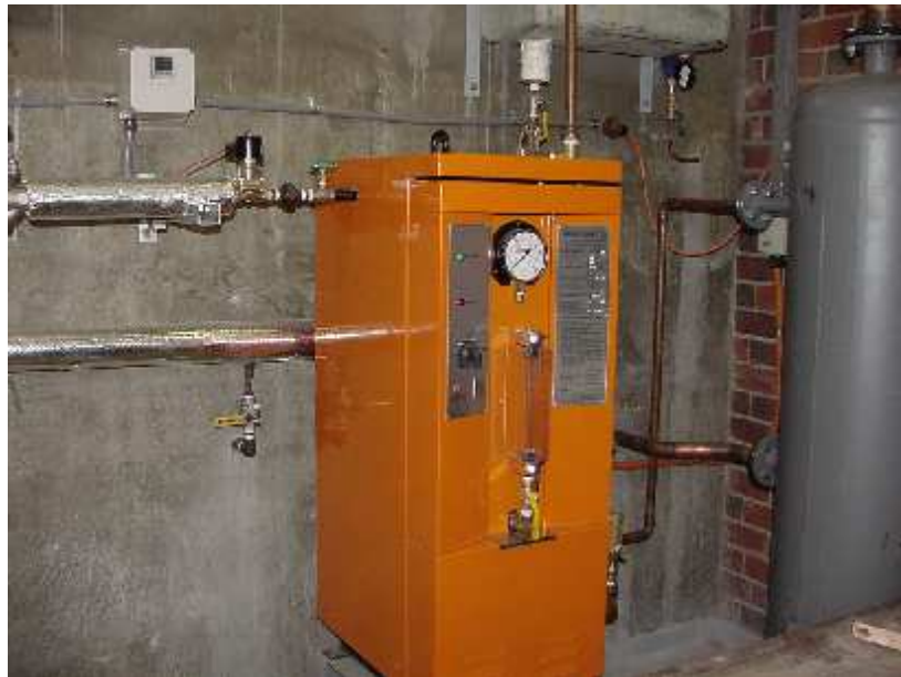
Figure 3.13: Steam Boiler and Controls
