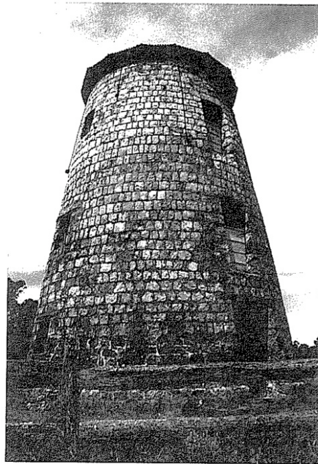
Figure 5 Erected in the 1830s, Chapman's Mill at Busselton is one of only a small number of early colonial buildings in this area listed on the Western Australian Heritage Register, as places must be of significance to the 'State' in order to meet the threshold.
