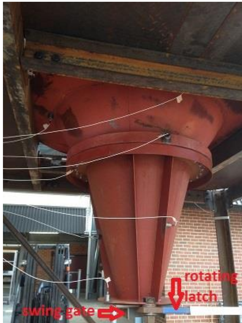
Figure 4-9: 200 mm hopper opening with swing gate in locked position.
