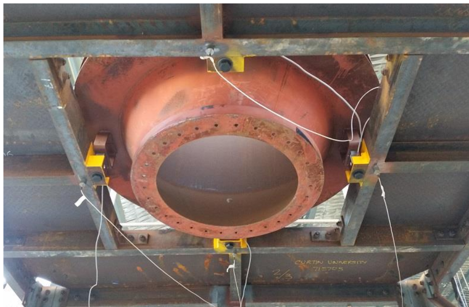
Figure 4-21: Silo supported on 4 x load cells – Bottom View.
