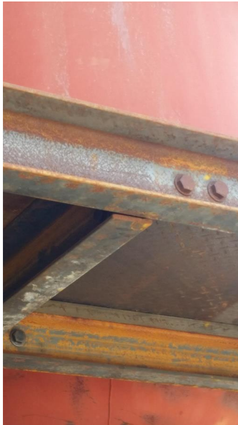
Figure 5-17: Damage to test silo support structure due to silo quaking.
