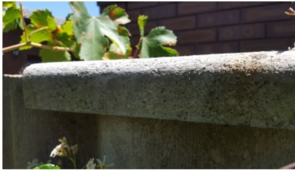
Super Six fencing with asbestos cement capping
