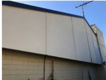
Flat asbestos cement sheeting used for external wall cladding above the brick.
