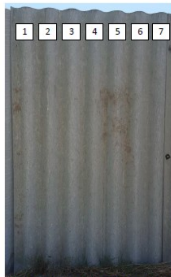
Super Six (right) contains asbestos and has 7 ridges per panel.
