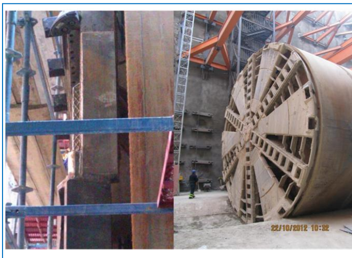
Fig. 8 Original gap between the shield and cutterhead of EPB-TBM
