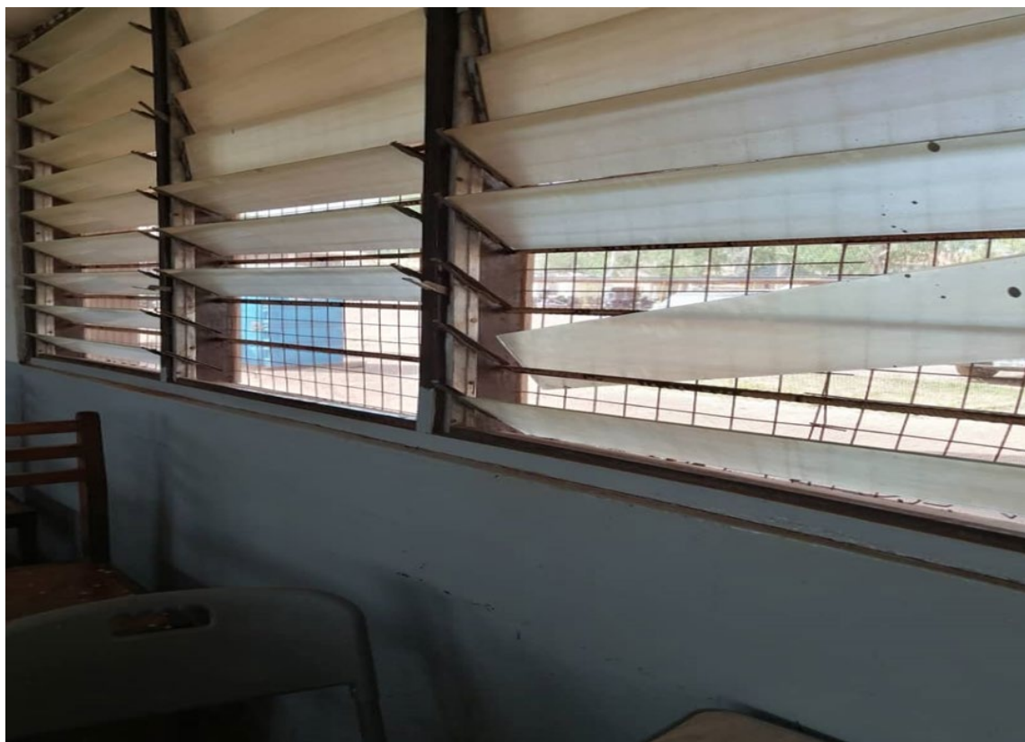
Figure 6-4: A lecture hall with broken louvre blades.
