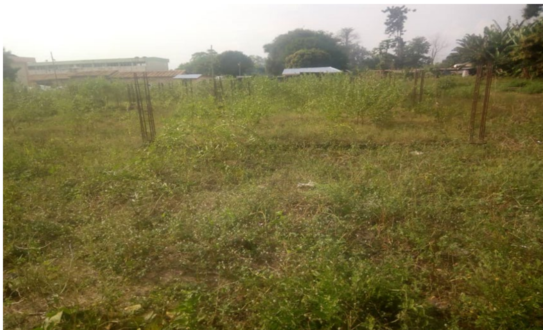
Figure 7-3: Staff office accommodation abandoned at foundation stage
