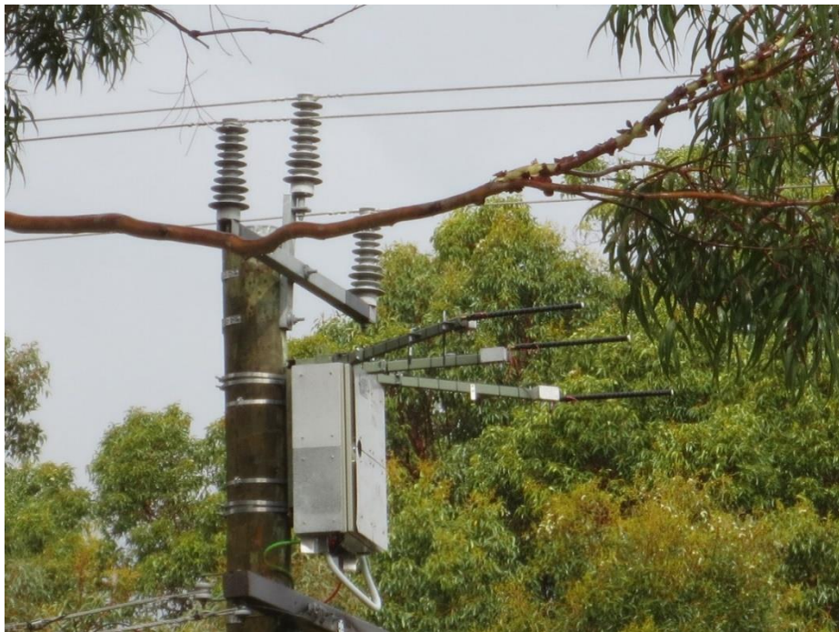
Figure 10.12. The travelling wave detector prototype installed on the medium voltage distribution network.
