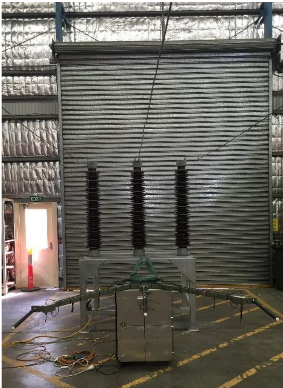
Figure 10.9. The equipment under test at the Western Power high voltage laboratory.
