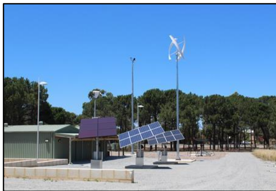
Figure 5-16 - GEEP facility- Curtin University Bentley Campus [99]
