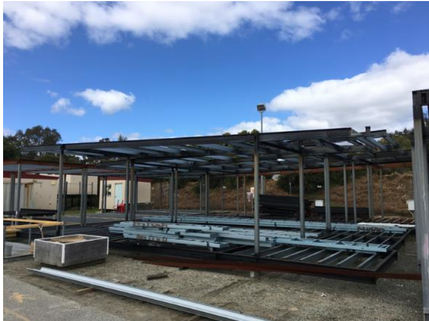
Figure 4.1 – Image of the frames in the Modular builders’ yard (2018). This frame served as the muse for what was to come (picture by author).
