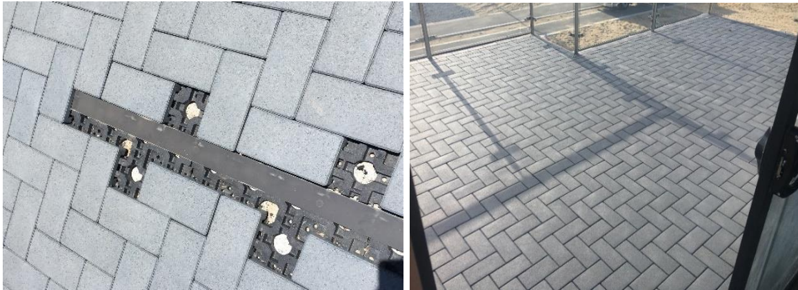
Figure 5.14 – (a) a plan view of the finished silo flashing (b) the finished balcony with the flashing design hidden by the recycled interlocking paving system
