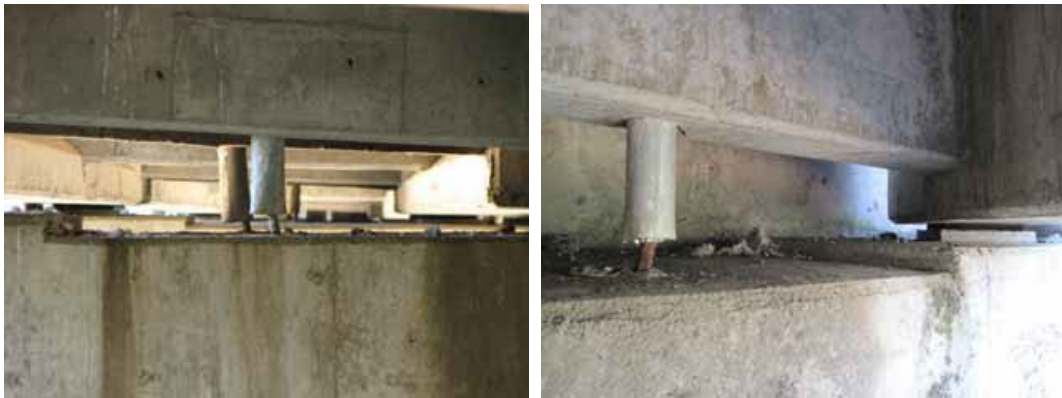
Figure 7. Metallic yielding dampers on Chilean bridges (after Elnashai et al. 2010)
