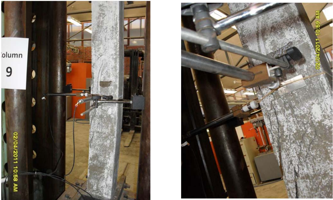
Figure 4.9: Failure mode of column GCIII-C3: (a) column after failure; (b) closer view of failure section
