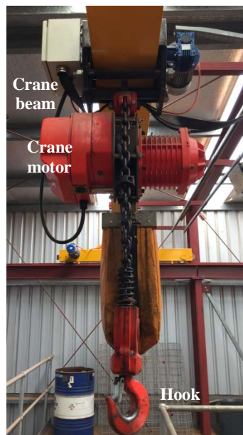
Figure 27: The overhead crane arrangement.
