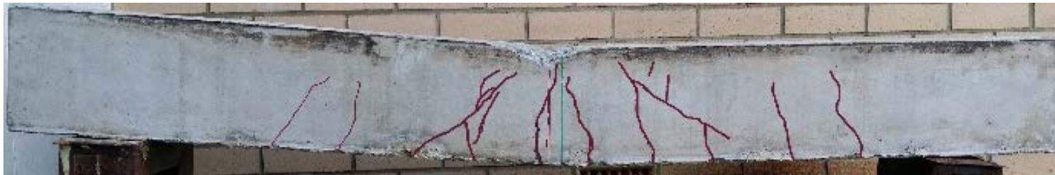
(b) Failure of the RC beam after testing
