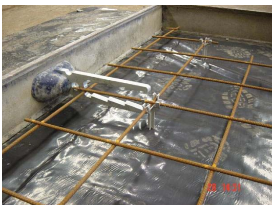
(c) Series 3 Test Panel prior to installation of perimeter bar with SL82 mesh
