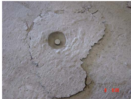
Figure 5. Panel of Series 7 with failed footed anchor
