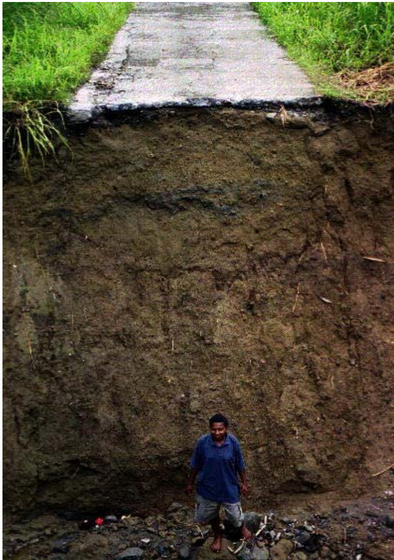
Plate 2.1. Collapsed culvert at Igora VOP, Popondetta
