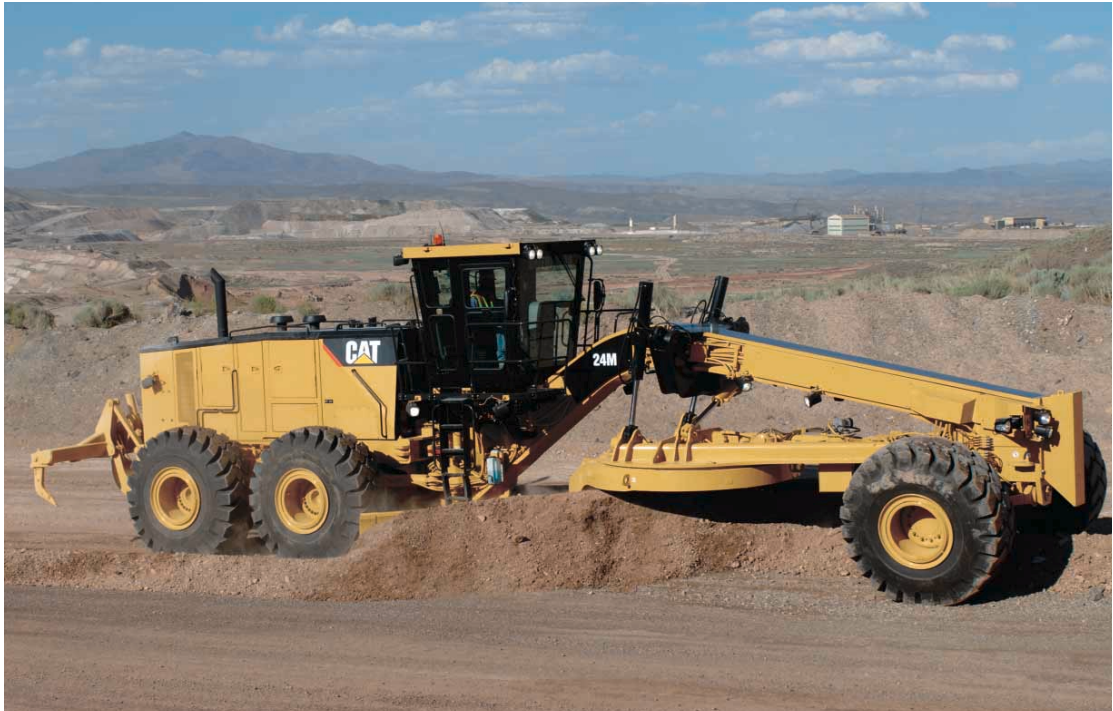
FIGURE 1.6: A grading machine smoothing the road for the trucks to reduce the effect of rolling resistance (CAT 2007).
