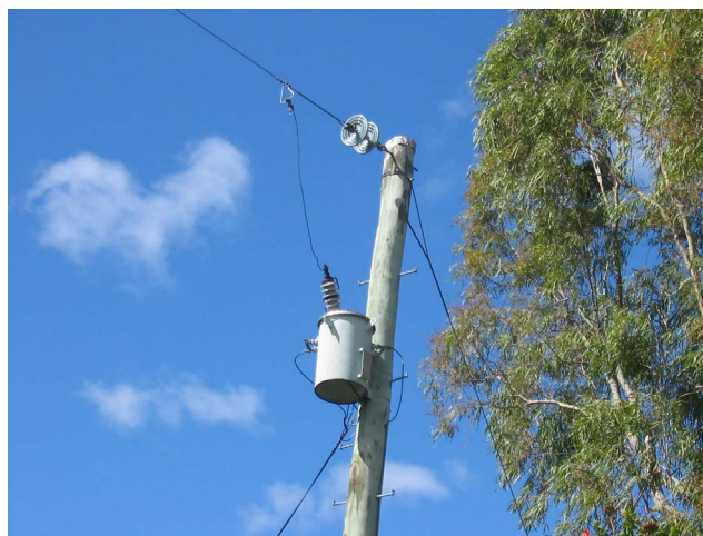
Fig 1. A SWER Customer Transformer, [8].
