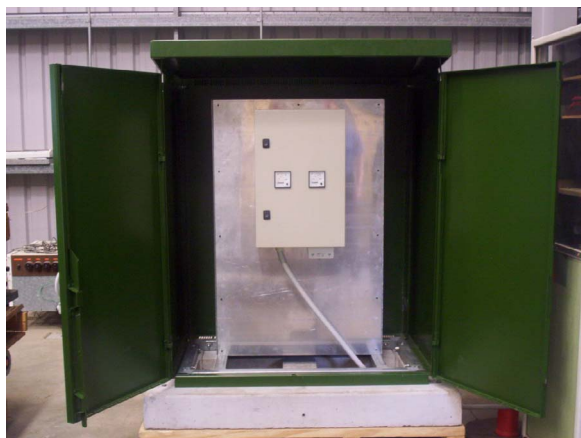
Fig16. SWER Voltage Controlled Reactor System
