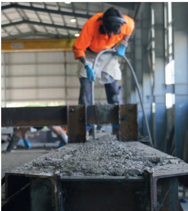
Figure 7: EFC geopolymer concrete being vibrated into the beam moulds at the Precast Concrete factory in Brisbane.
