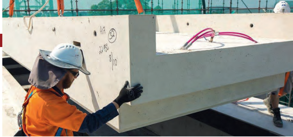
Approximately 30,000m 3 of EFC will be used for the Wellcamp Airport's taxiways and apron.
