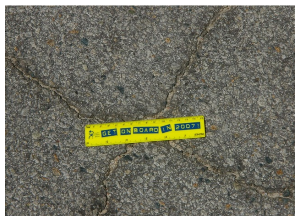
Fig. 3. Moderate severity block cracking.
