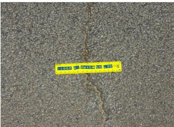
Fig. 6. Moderate severity transverse cracking.
