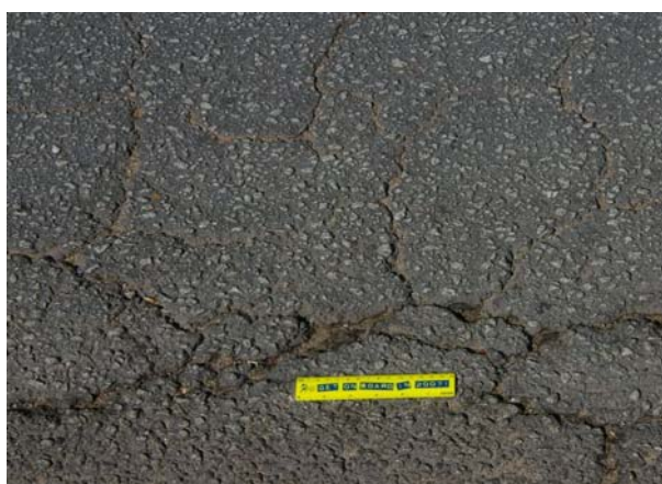
Fig. 2. High severity fatigue cracking.
