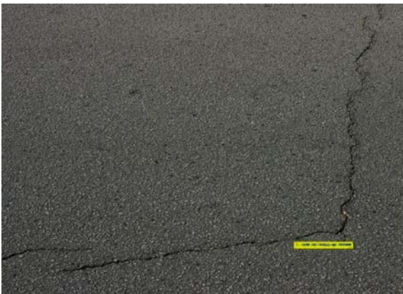
Fig. 5. Moderate severity reflection cracking.
