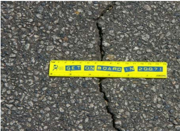
Fig. 4. High severity longitudinal cracking.
