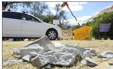
Figure 22: 'DANGEROUS SPLIT' (Item 65)
