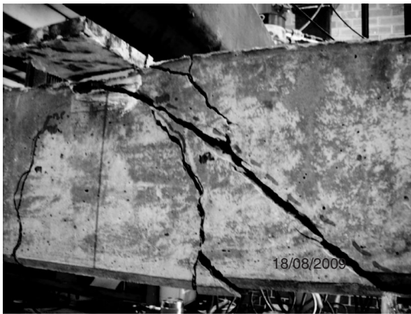
Figure 6. Typical shear compression failure
