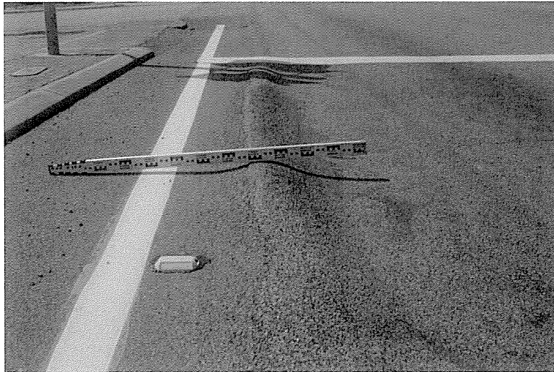
Figure 2.9: Shear failure at Bannister - Forum intersection.
