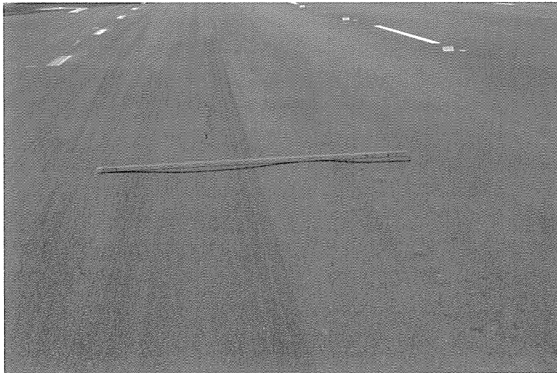
Figure 2.12: Shear failure Kewdale Dowd intersection 2012.
