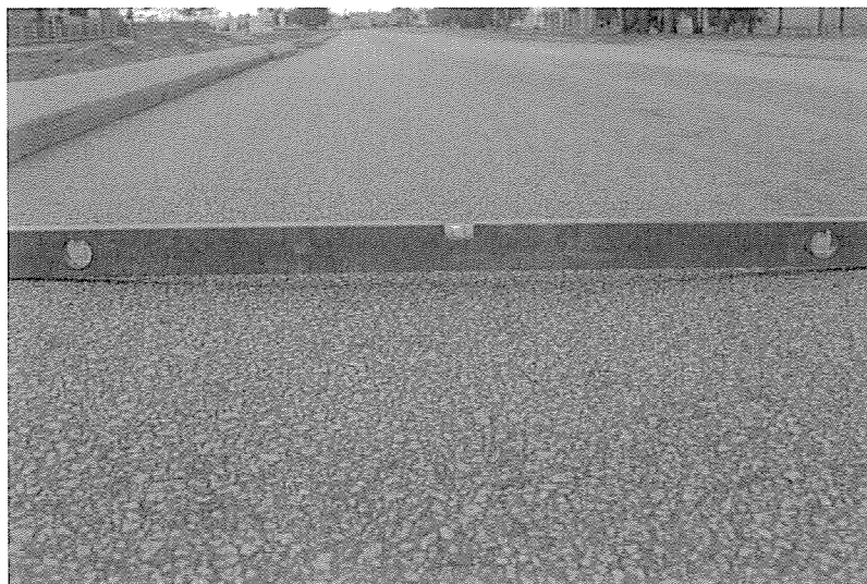
Figure 2.11: Shear failure Kewdale near Welshpool intersection 1999.
