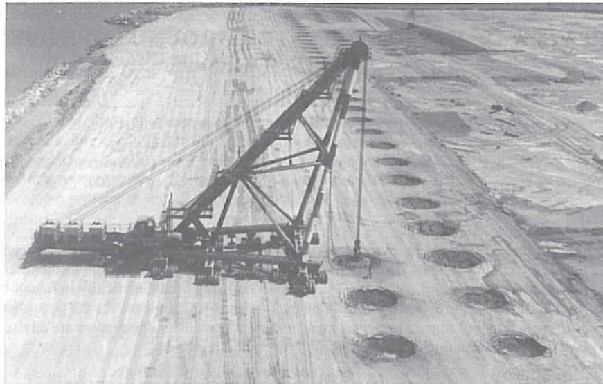
Figure 2: Menard Giga Machine lifting a 170 ton ponder at Nice International Airport (Menard).
