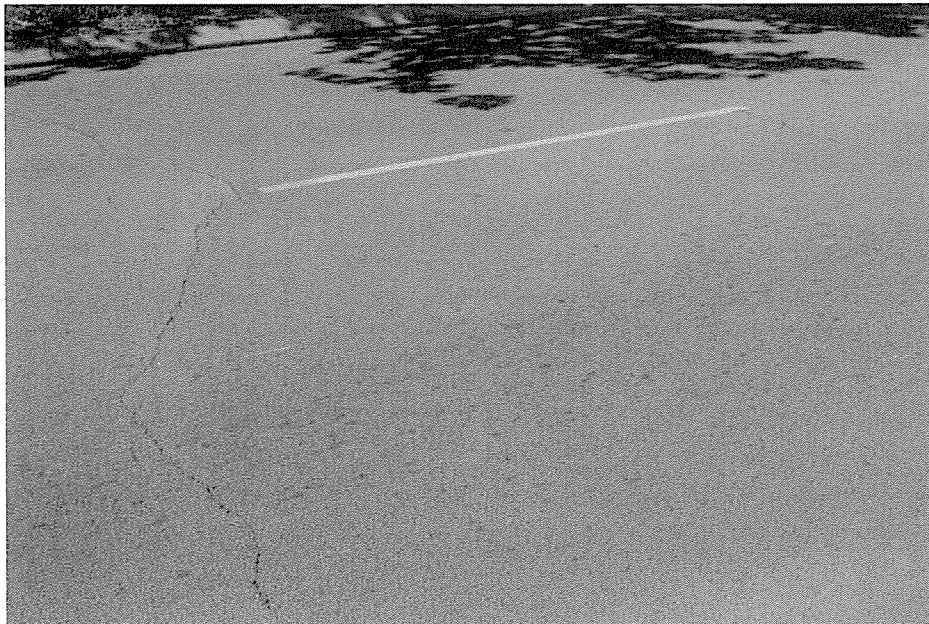
Figure 2.1: Transverse cracking in High Road.
