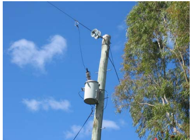
Figure 1: A SWER Customer Transformer
