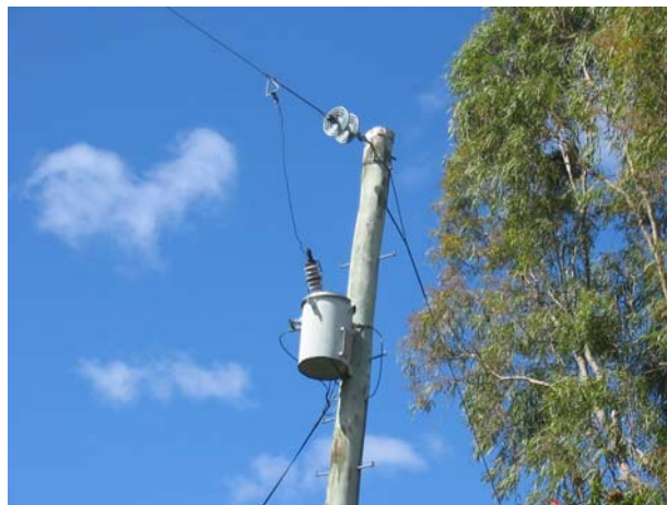
Figure 1: A SWER Customer Transformer, [4].
