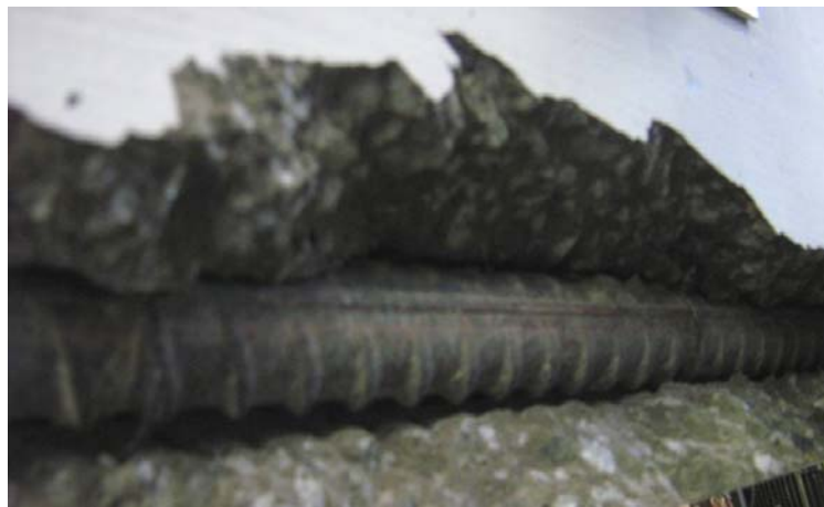
Figure 8.8: Surface Condition of Reinforcing Bars After Failure (Normal Strength Concrete – Beam N-L-30)
