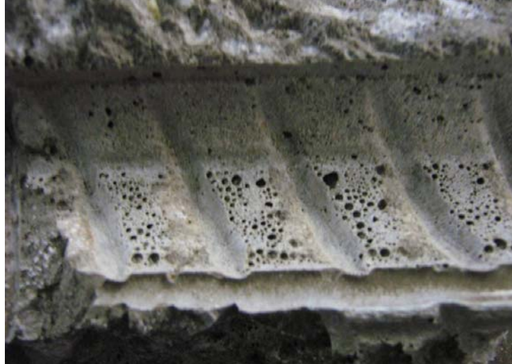
Figure 8.9: Rib Patterns of Bar on Geopolymer Concrete (Normal Strength Concrete – Beam N-L-30)
