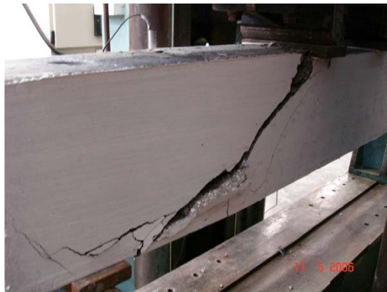
Figure 4.10: Principal Diagonal Crack for Beam S2-1
