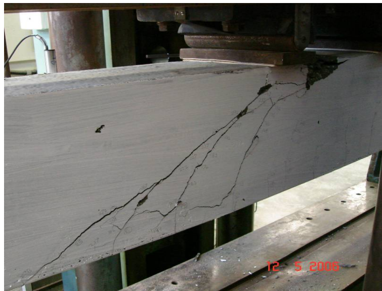
Figure 4.13: Concrete Crushing in Compression Zone for Beam S2-2
