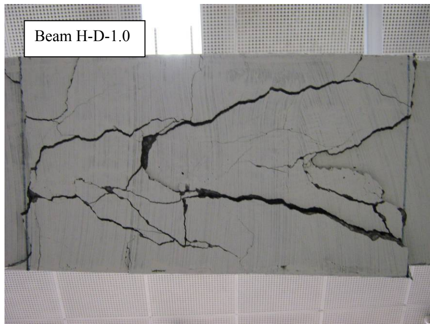
Figure F.7: Crack Pattern for Beam N-D-1.0 and H-D-1.0 (Bottom View)
