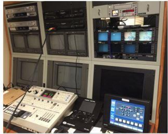
Control Room Workspace
