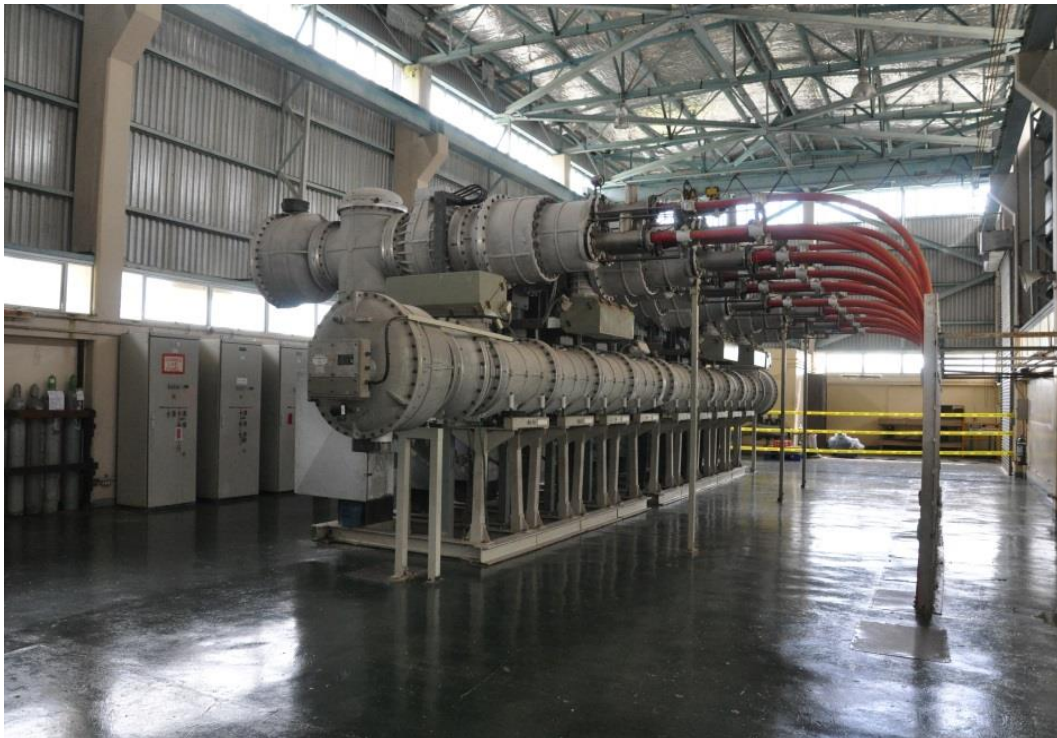
Figure 1. High voltage switchgears
