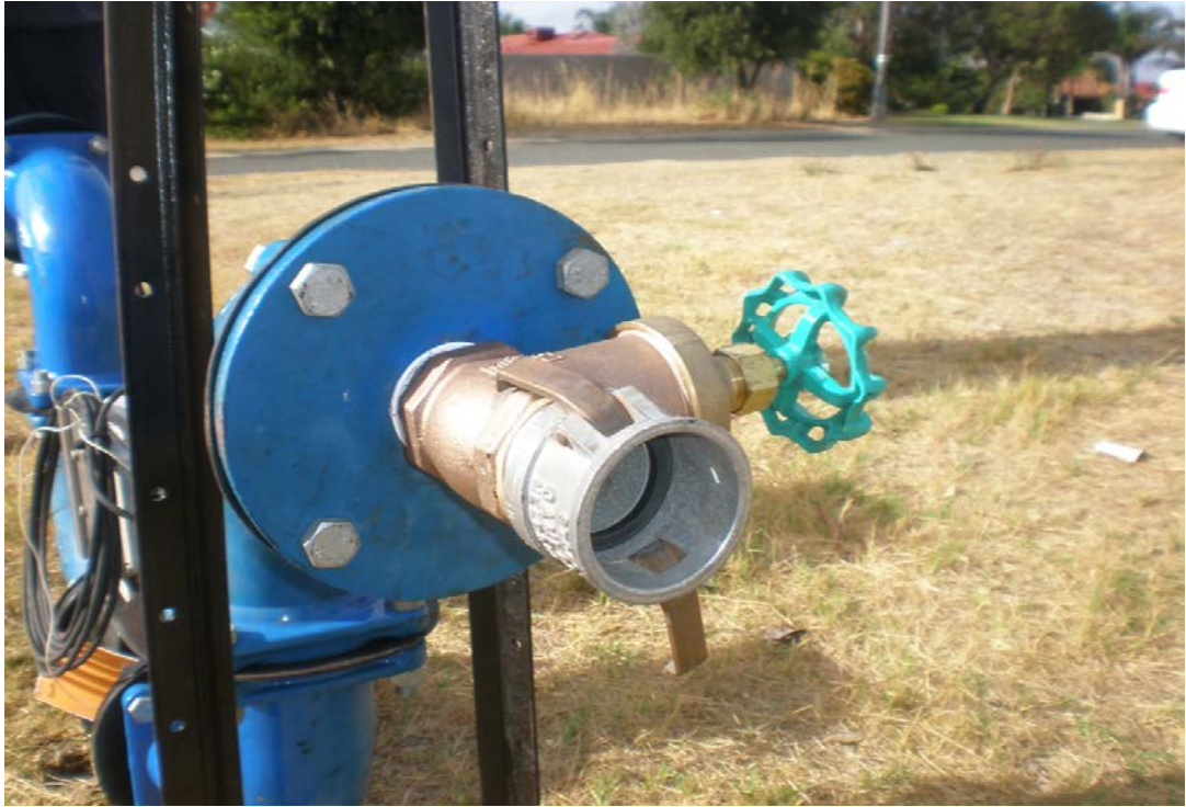
Figure 5.3: Control valve next to the flow meter.
