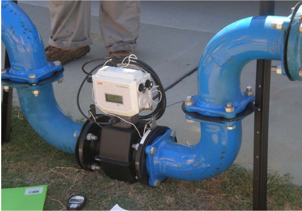
Figure 5.1: Flow meter connection with u shaped 100 mm pipes.
