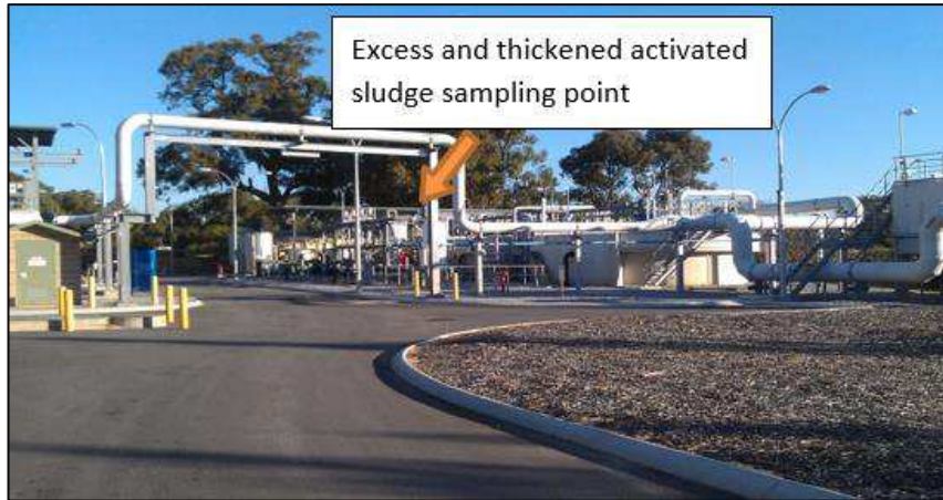
Fig. 4.1 Excess activated sludge and thickened excess activated sludge sampling point at Beenyup WWTP
