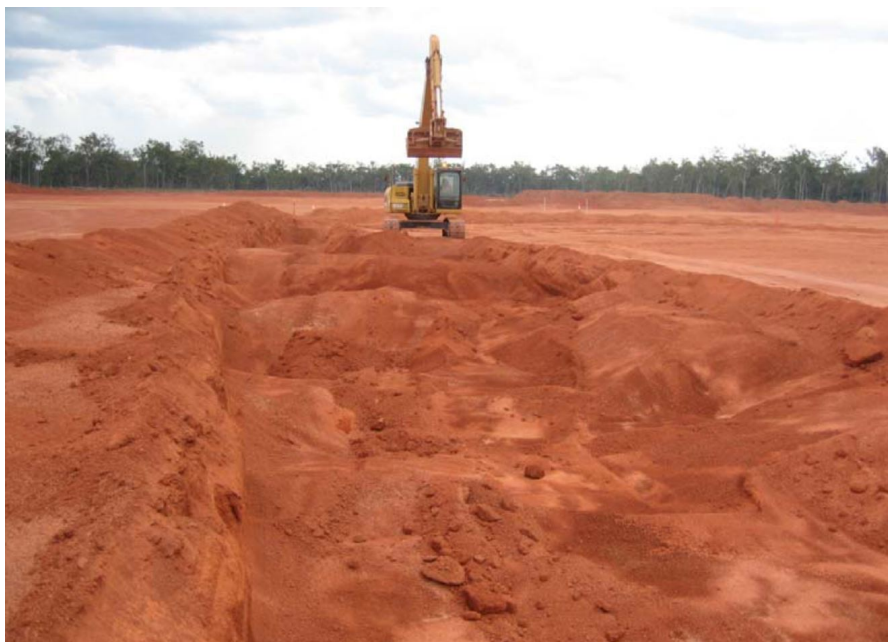
Figure 3.3: The test excavation conducted to reveal the characteristics of the lateral variability inherent in the geological interface (Erten, 2012)
