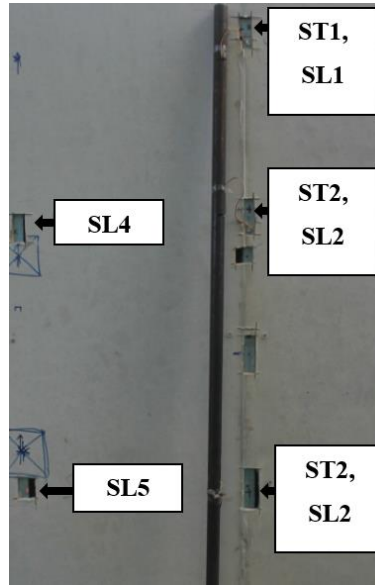
Figure 3.50: Southern Wall In-Situ Thermocouples
