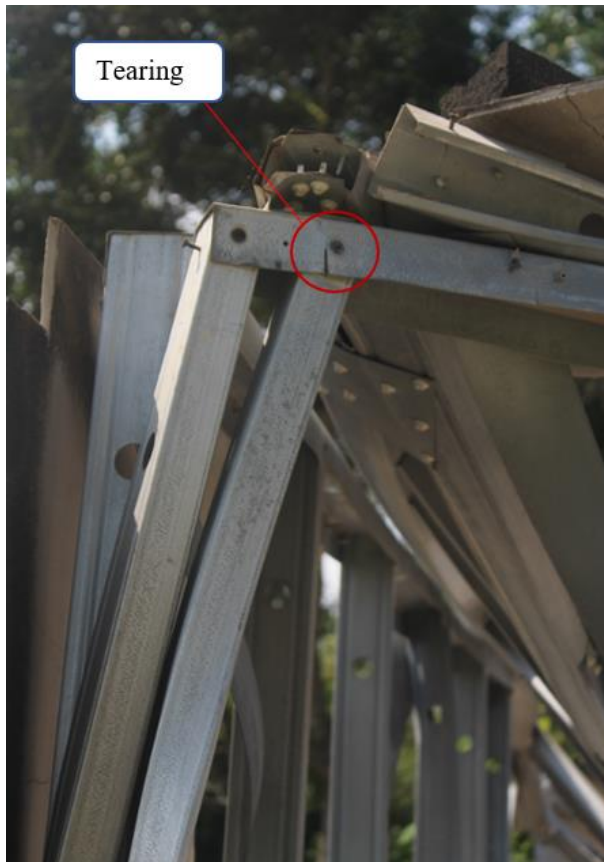
Figure 6.37: Tearing of Top Rail in North Wall
