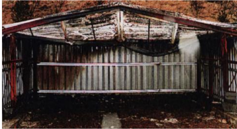
Figure 2.8: Asymmetrical Collapse (Wong, 2001)
