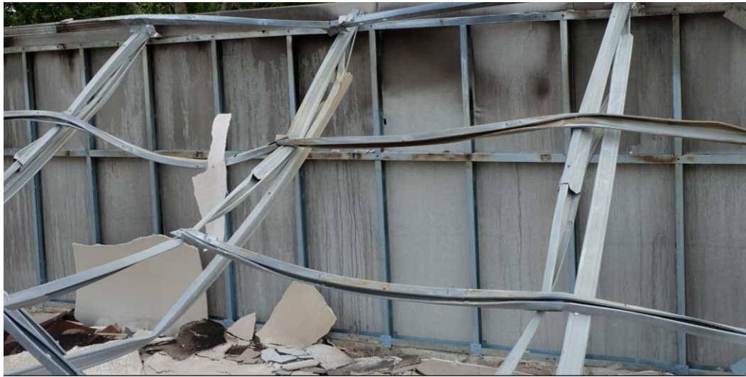
Figure 6.35: End of Full-Scale Fire Test at Southern Wall
