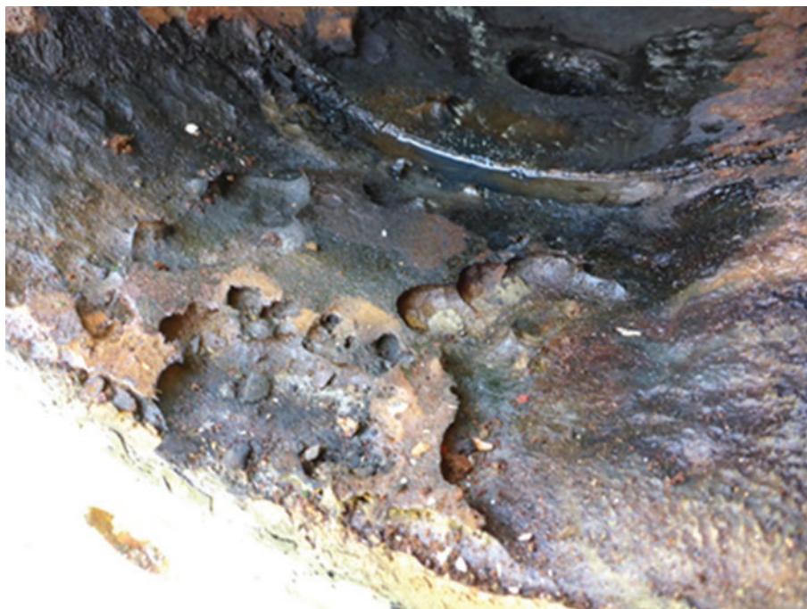
Figure 3. Microbiologically influenced corrosion of crude line to cargo storage (0.5% water cut).
