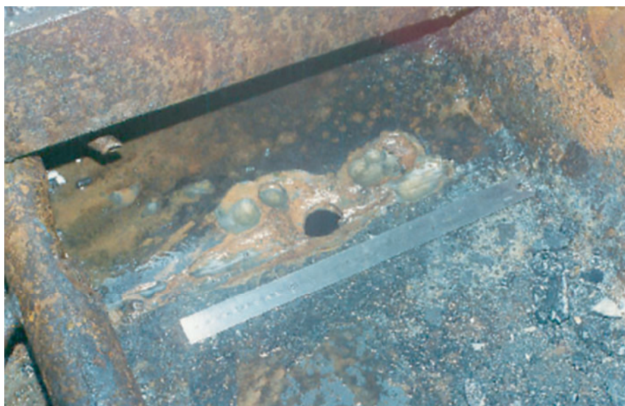
Figure 2. Microbiologically influenced corrosion of high pressure separator horizontal baffle.
