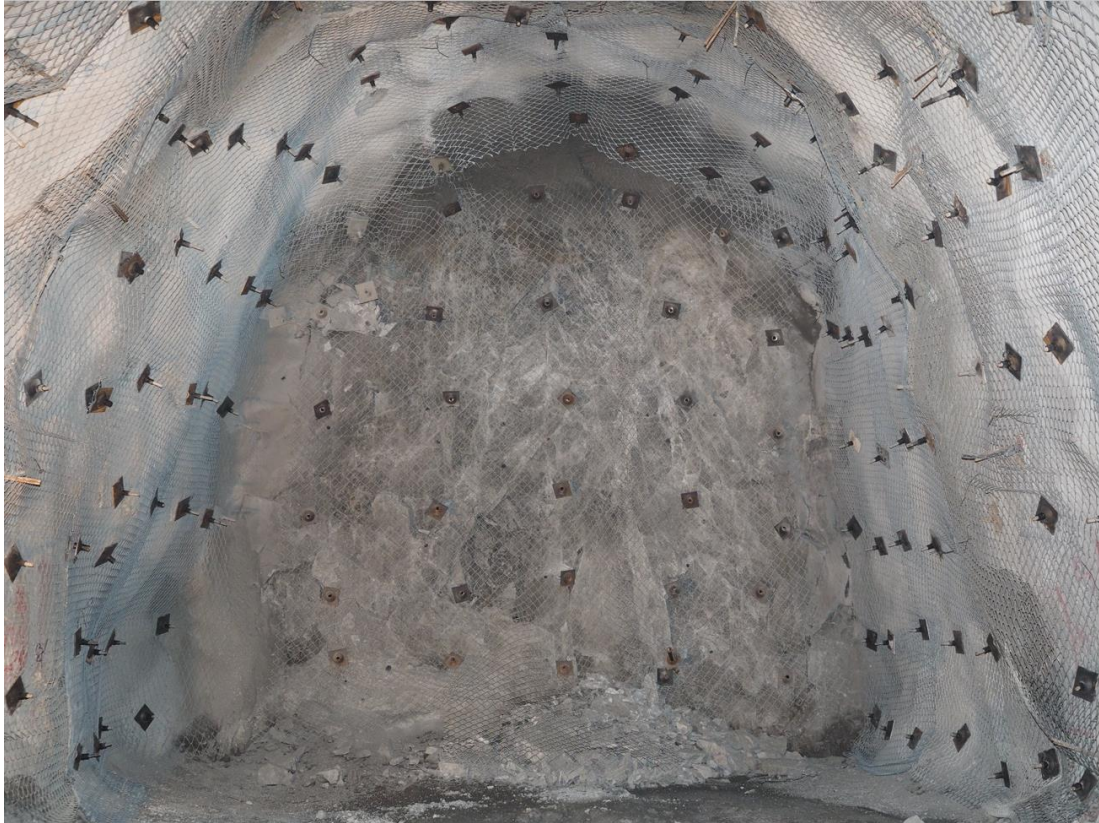
Figure 206 - Temporary face support to contain face instability during drill and blast activities.
