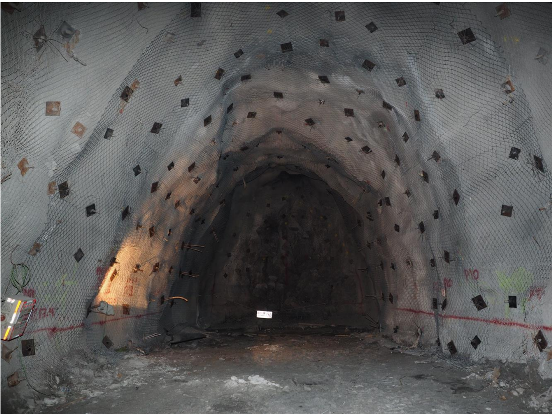
Figure 223 – Multi-layered, high energy dissipation ground support scheme installed in the north tunnel.
