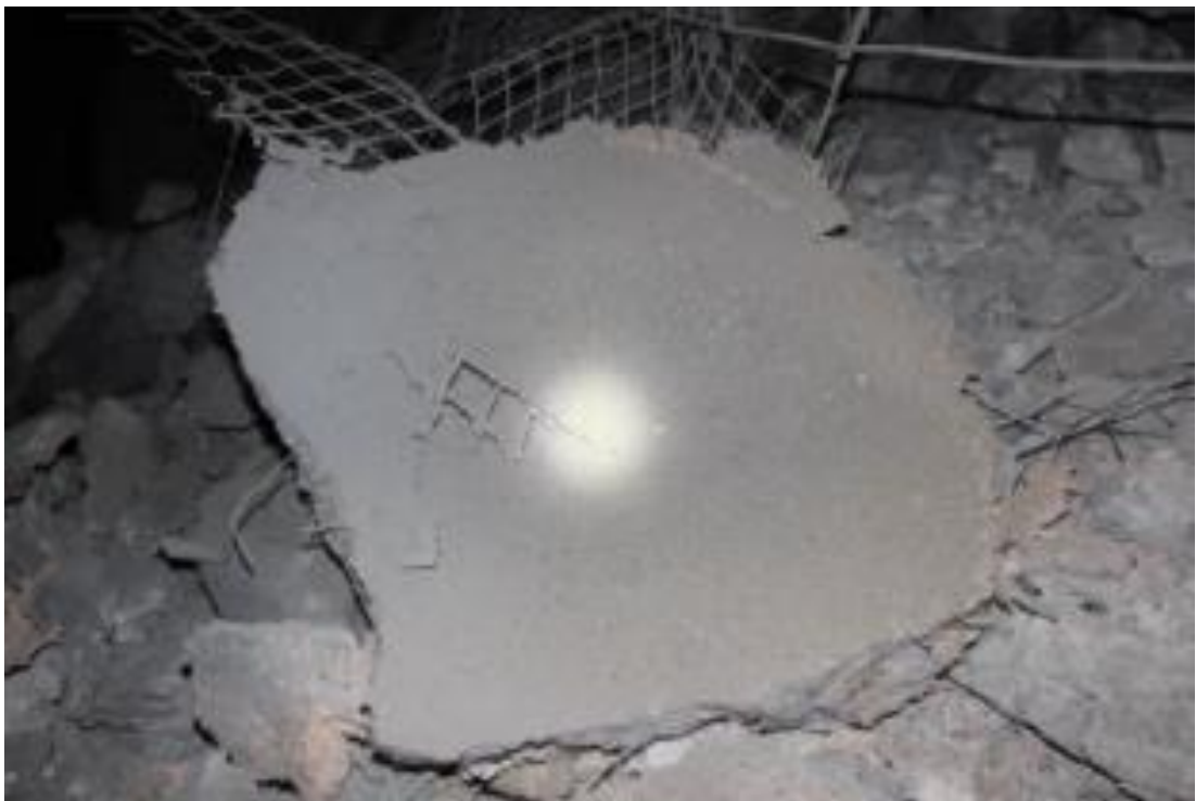
Figure 48 - Mesh-reinforced shotcrete failure in large blocks due to high energy demand (Drover, 2014).
