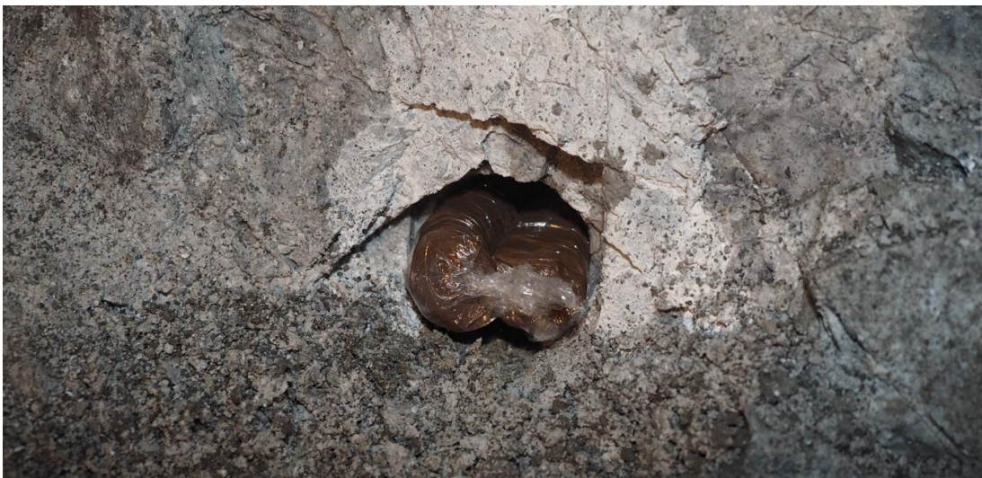
Figure 183 - Damp clay stem packs inserted into the destressing borehole prior to tamping.
