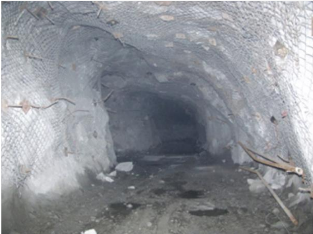
Figure 15 - Example of notch formation due to stress-driven brittle failure in an underground tunnel.
