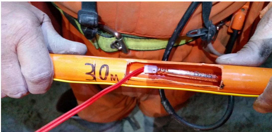
Figure 247 - Detonators were inserted into the boreholes at specific lengths using rigid conduit.
