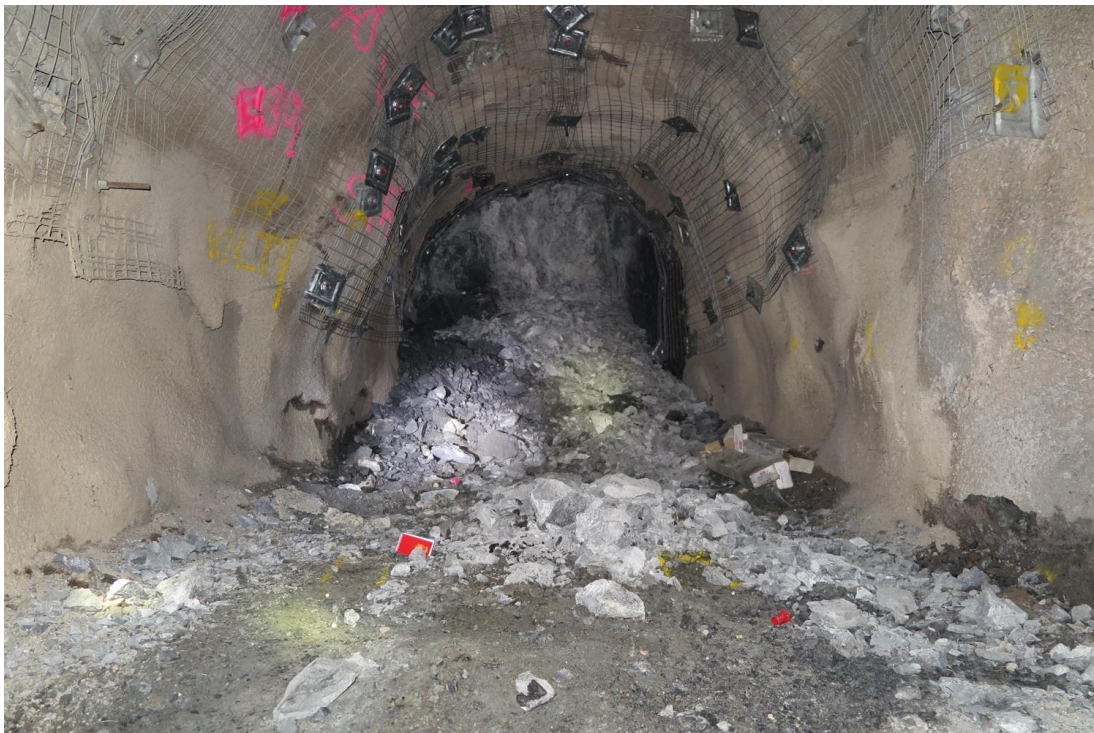
Figure 170 - Violent stress-driven failure causing ejection of rock from the development face.
