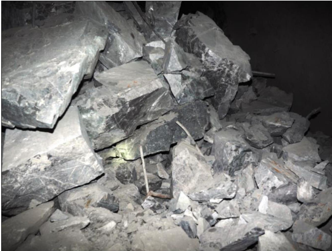
Figure 103 – Reinforcement and surface support failure, with ejection of large blocks.
