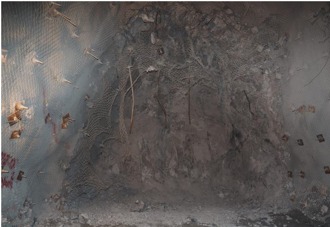
Figure 186 - Damaged temporary face support required to be removed following blasting.
