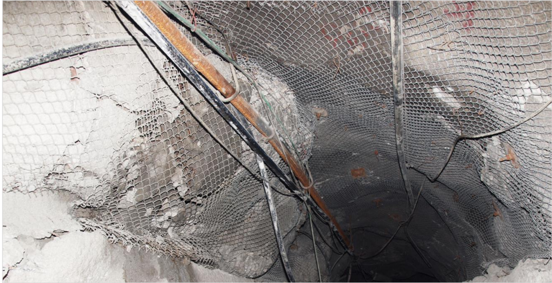
Figure 156 - Large displacement of external woven mesh connected to adjacent stable reinforcement.
