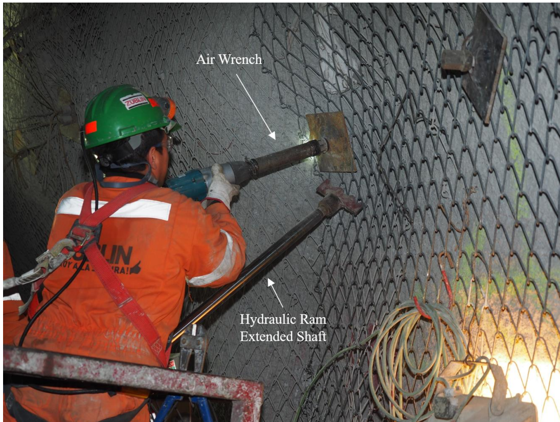
Figure 218 - Use of a hydraulic ram to install mesh and second plates on the primary reinforcement.
