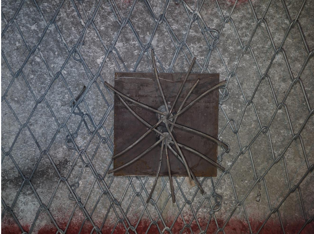
Figure 219 – Unfurled cable strands at the external fixture.
