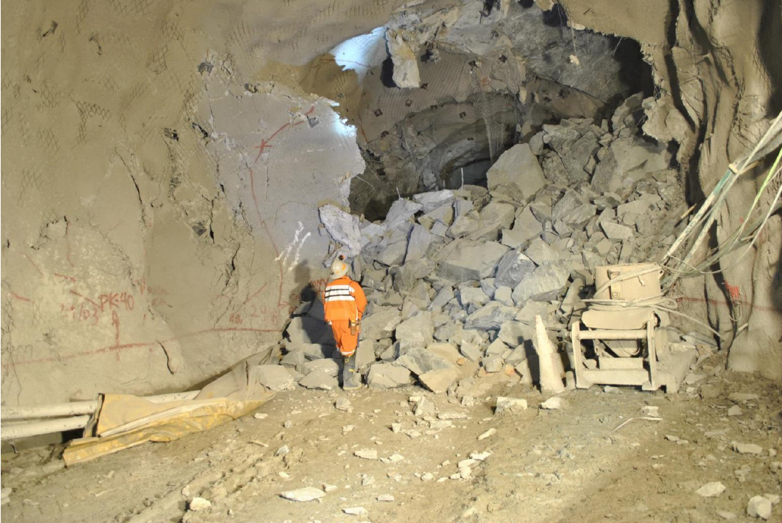
Figure 208 - Structurally controlled excavation failure more than 20m from the development face.
