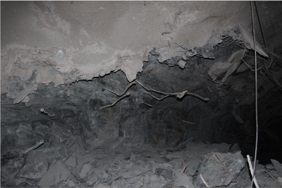
Figure 31 - Violent fault rupture causing severe ground support damage.
