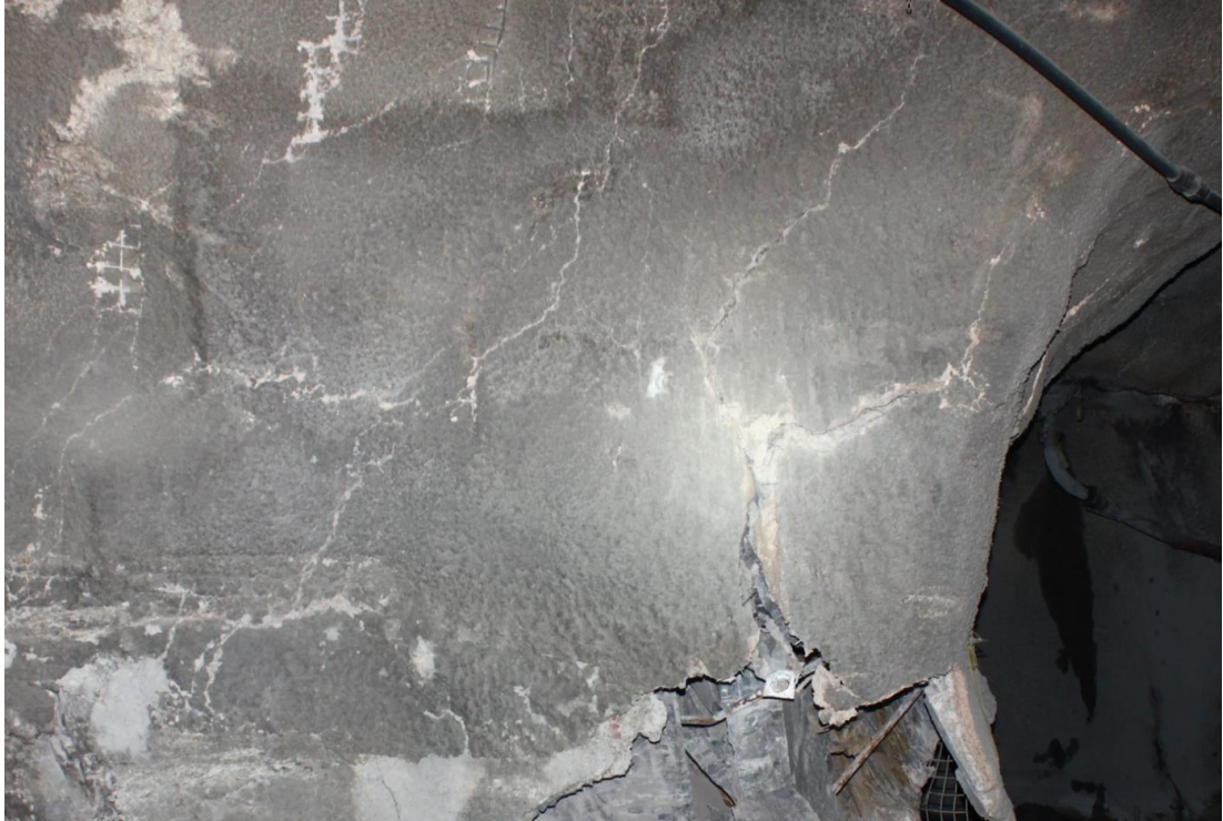
Figure 47 – Regular damage patterns in mesh-reinforced shotcrete after violent loading (Drover, 2014).
