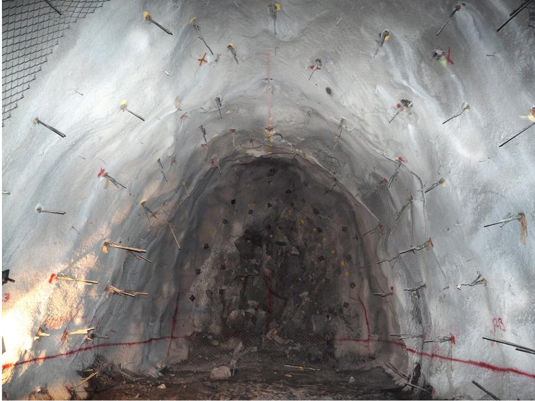
Figure 212 - Secondary reinforcement installed awaiting the second layer of high capacity woven mesh.
