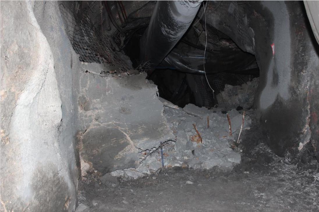
Figure 30 - Fault rupture causing severe excavation damage, with very high ejection velocity of instability.
