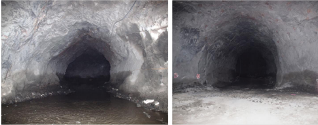
Figure 17 - Spalling failure of unsupported semi-circular tunnels at the roof (Villaescusa, et al., 2016b).
