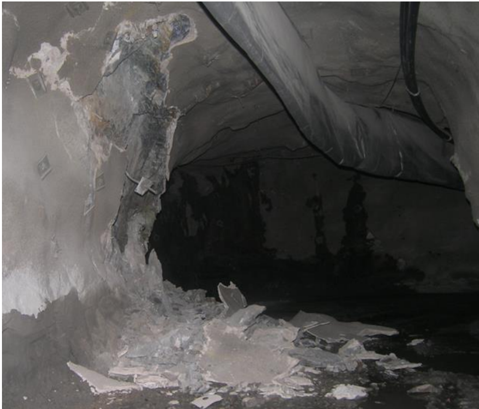
Figure 9 - Lack of ground support retention following a violent spalling failure of the excavation surface.
