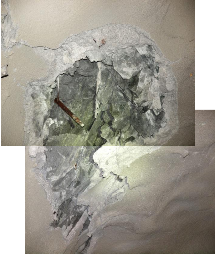
Figure 102 - Example of spalling failure with a shallow depth of instability.
