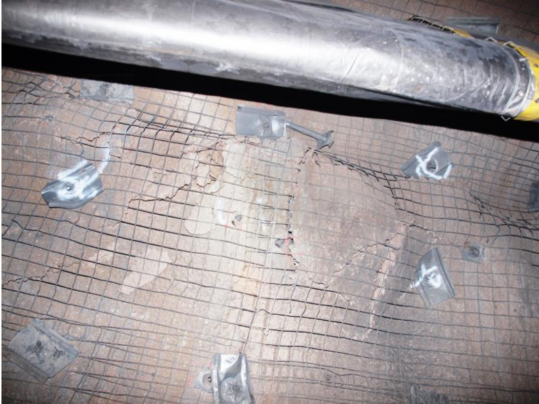
Figure 49 – Shotcrete failure prior to significant mesh loading (Drover & Villaescusa, 2015a).
