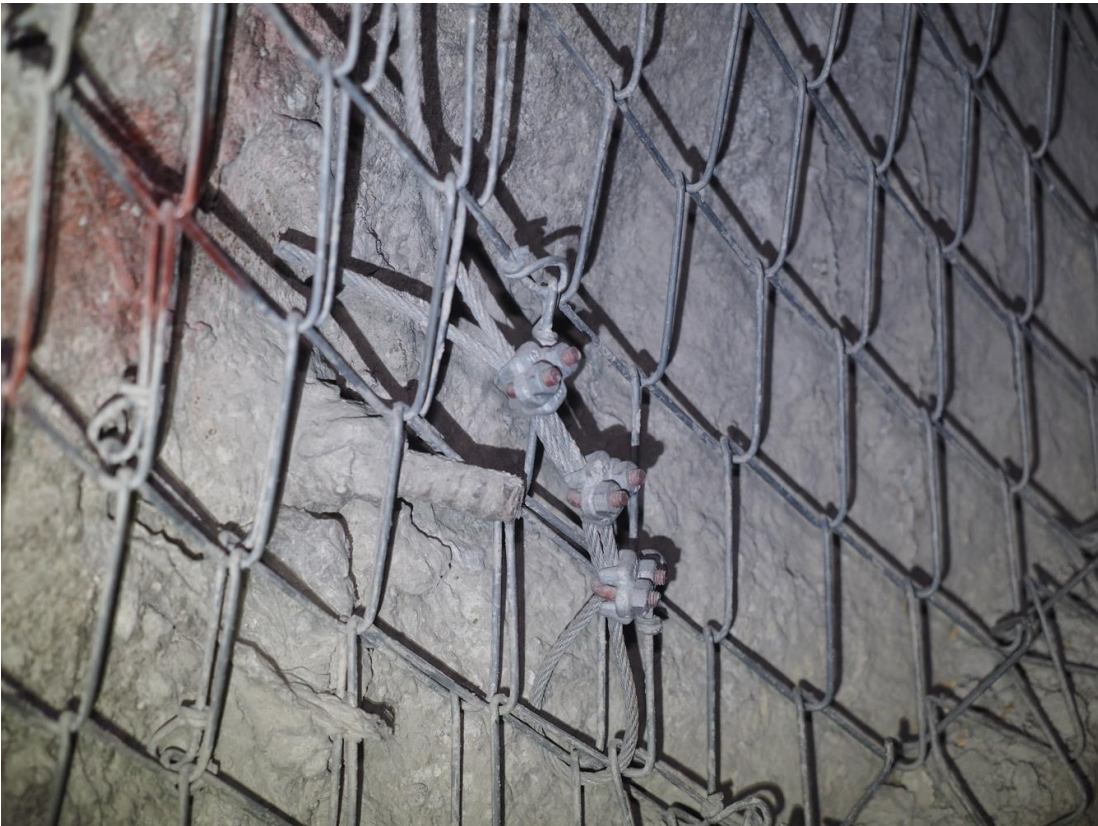
Figure 221 - Wire stitching through mesh sheet overlaps terminated with three crimps at floor level.
