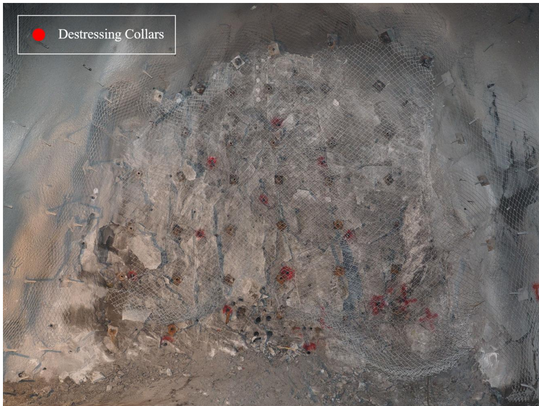
Figure 178 - Typical face conditions requiring minor remedial scaling behind mesh prior to charging.
