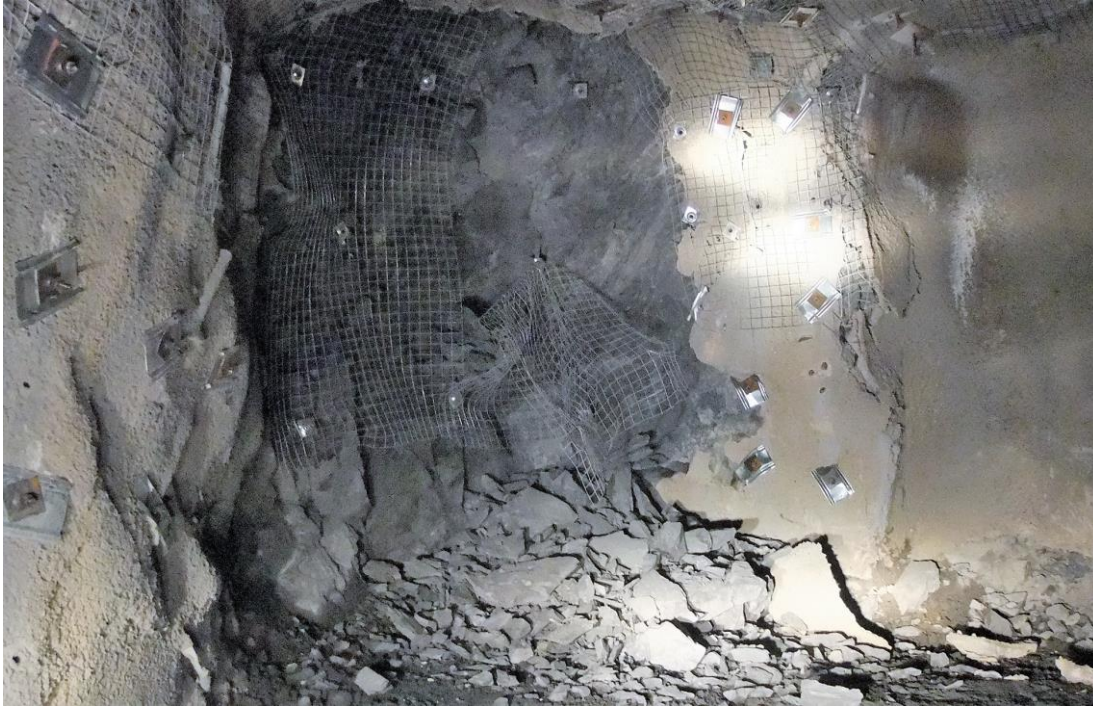
Figure 52 – Failure of temporary face support due to violent stress-driven instability.
