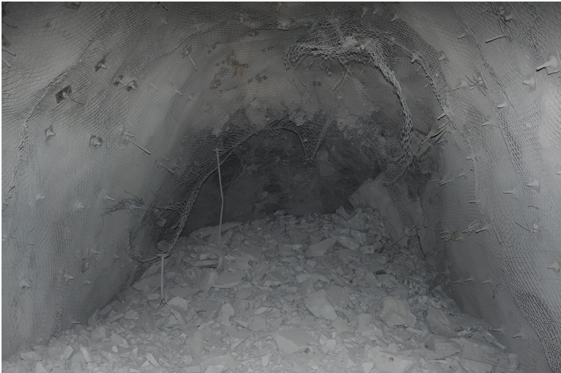
Figure 185 – Development blast rock and damaged temporary face ground support to be removed.
