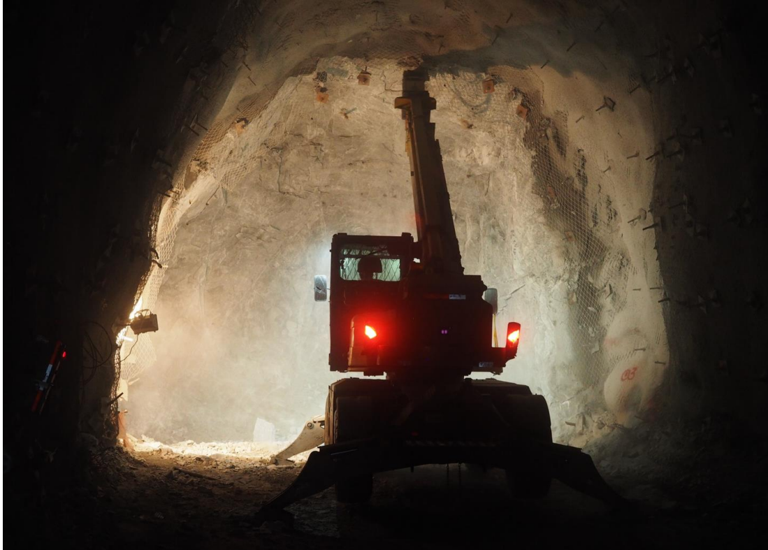
Figure 188 - Mechanical scaling of loose rock from the tunnel walls prior to shotcreting.
