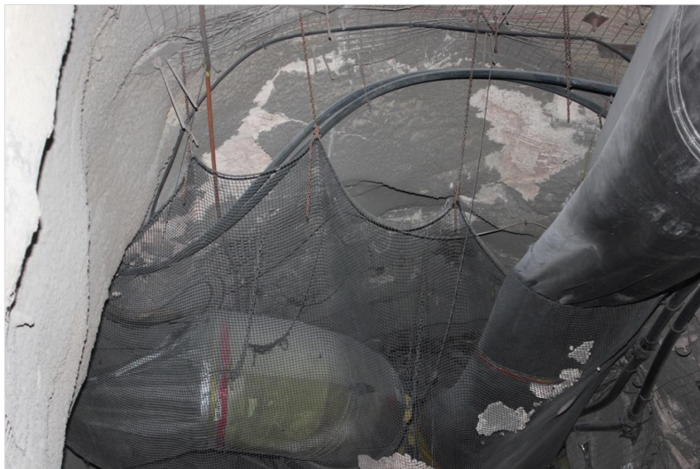
Figure 158 - Failure of an exposed mesh-reinforced shotcrete layer due to violent spalling.
