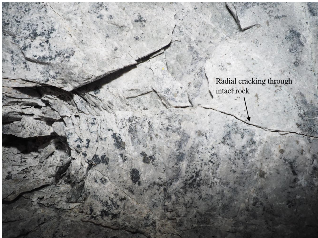
Figure 327 - Close-up view of destressing blast-induced radial fractures through intact rock.
