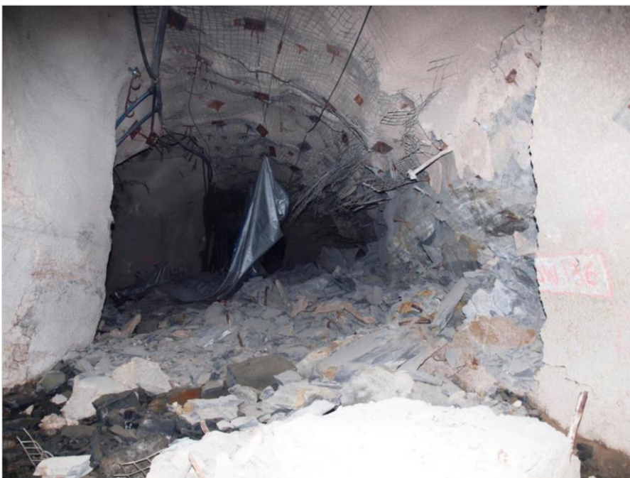
Figure 19 – Fault rupture mechanism of excavation instability causing extreme damage (Drover, 2014).
