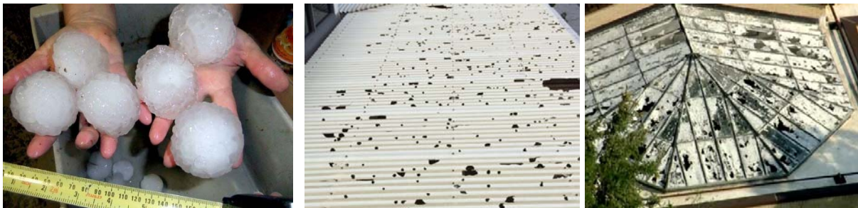
Fig 1: (L) Large Hailstone [20]; (M) Hail damage to roof; (R) Damage to roof panel [21].
