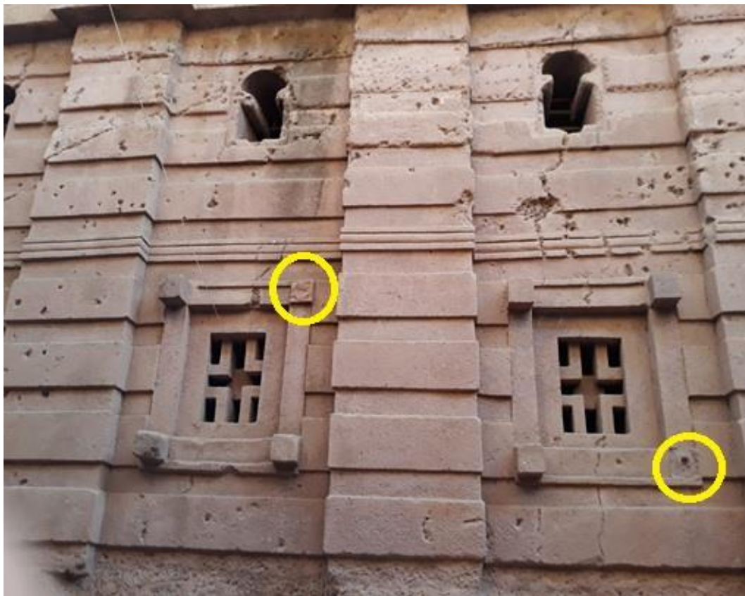
Figure 10: Monkey-head style protruding beams on Bete Amanuel. Severed beams (circled) were broken during the shelter construction.
