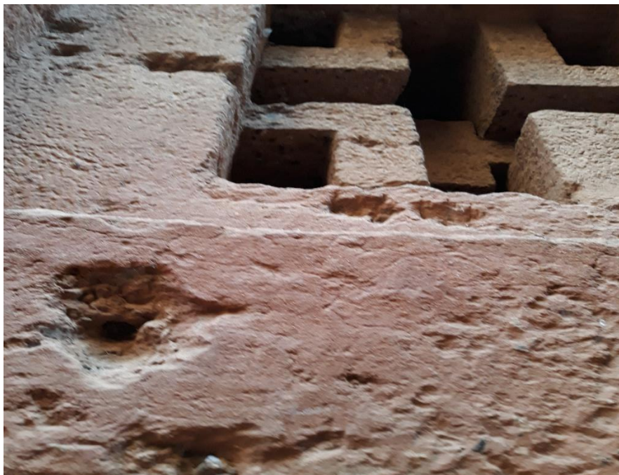
Figure 4: Close up of pockmarks on Bete Amanuel caused by nails.
