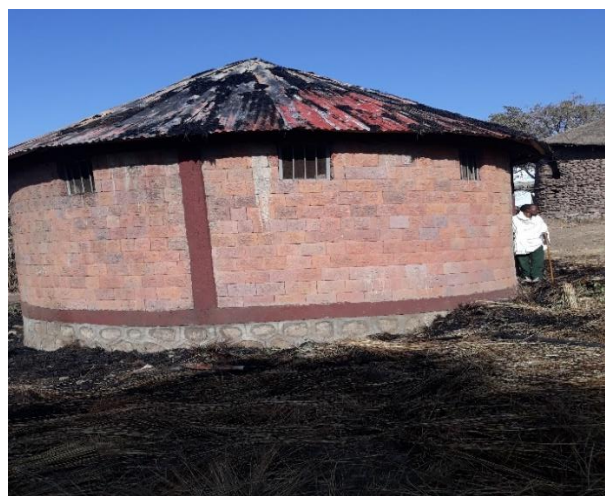
Figure 1: Burnt remnants of non-operation World Bank toilet, set on fire in January 2018.
