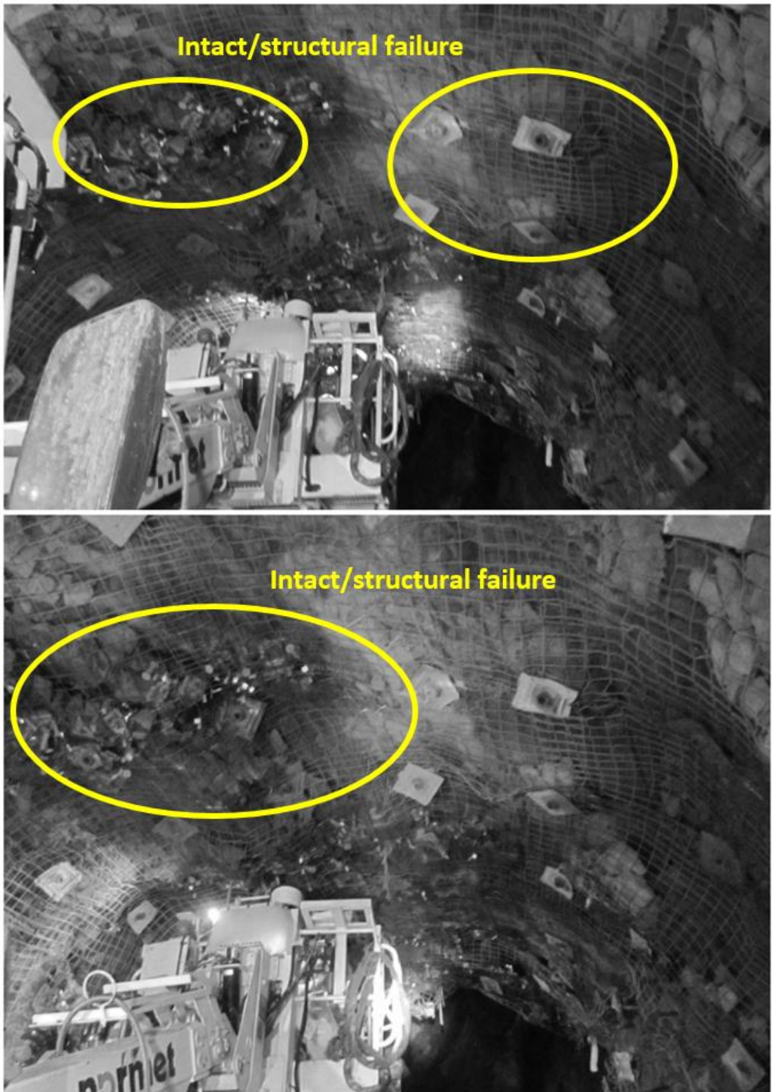
Figure 4.26. Ground problems in the decline and installed support devices
