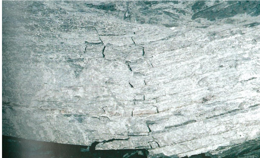
Figure 2.17. Roof fall in a mine (Peng, 2007)
