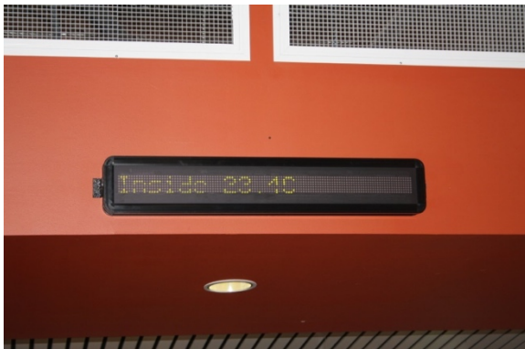
Figure 5.14: Temperature display controlled by the BMS at Amity PS
