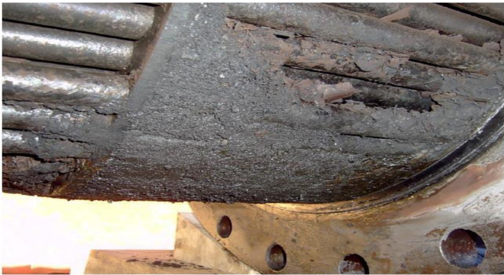
Figure 2-22: MEG Regeneration Kettle re-boiler tube bundle \text{FeCO}_3 fouling [64]
