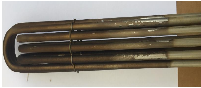
Figure 6-10: Scale formation on the heater bundle of the reboiler
