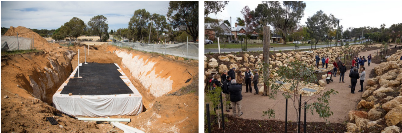
Figure 4. Left: installation of drainage cells as part of the retrofitting of the stormwater sump; right: the completed stormwater sump with a newly landscaped parklet for community use. Source: LandCorp (2015).
