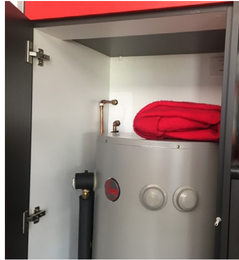
Fig. 5. Use of heating pump space as a drying or freshening cupboard by SHAC resident J with a blanket in the cupboard to freshen up and improve the smell.
