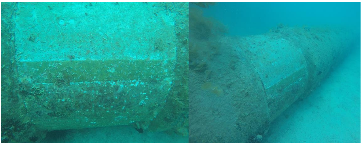
Figure 6-8: Anodes in the proximity of the crossing point.
