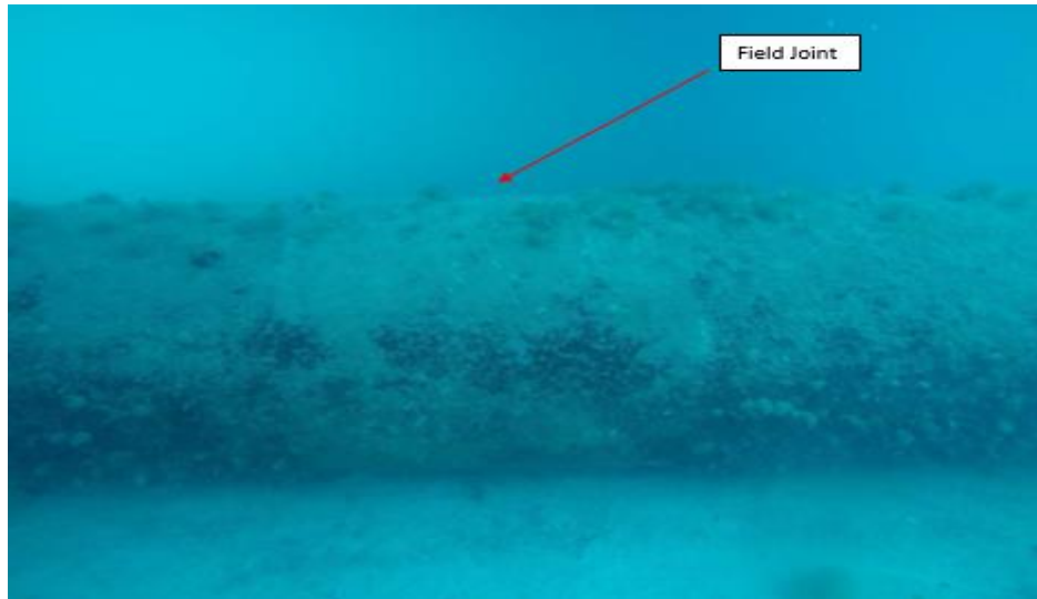
Figure 6-29: Field joint coating downstream from the damaged joint- Pipeline # 1.
