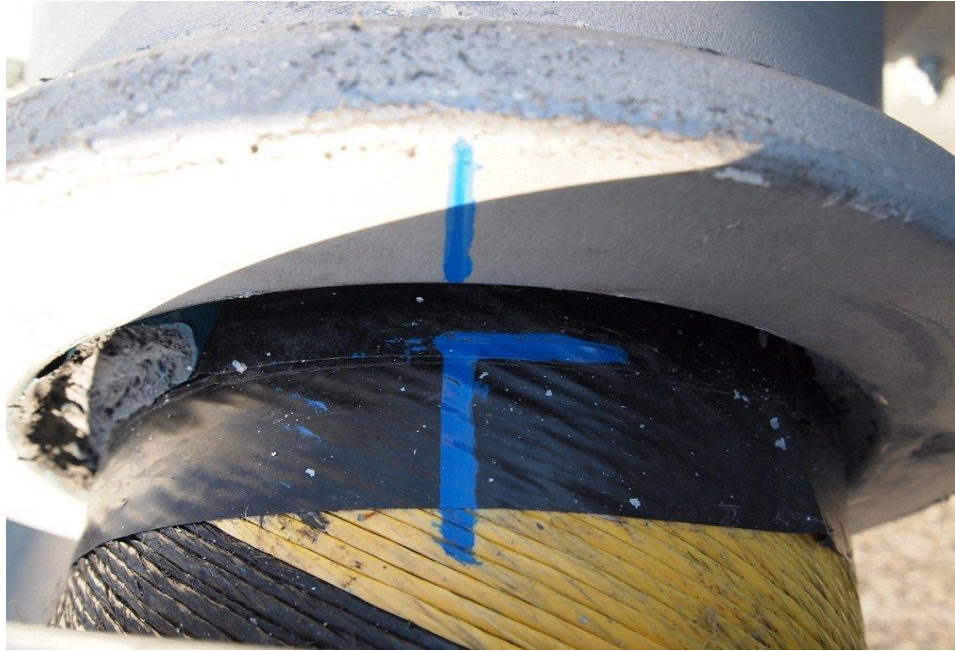
Figure 5-21: Marking on cable.
