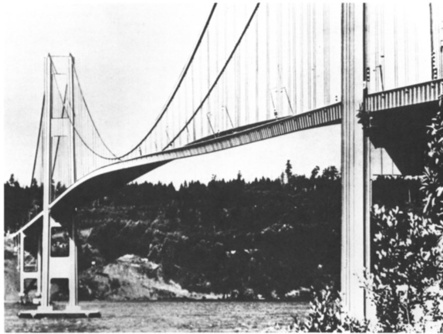
Figure 1.1: Photograph reproduced from Gunns (1981) showing the flow-induced vibrations of the Tacoma Narrows Bridge: “The writhing motion of the bridge deck was caused in part by wind action on the solid sideplates. (James Bashford, Photography Coll., University of Washington Libraries)” (Gunns, 1981).
