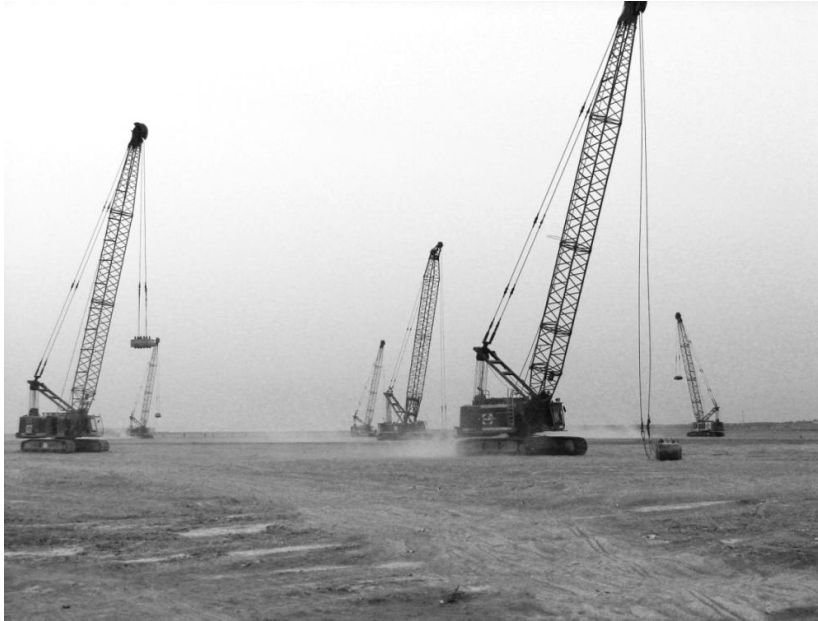
Figure 3. Implementation of 11 special cranes for DC (not all shown in this picture)
