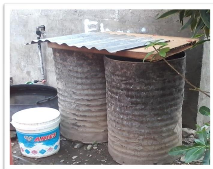
Figure 22: Informal Unkept Water Infrastructure -Domestic Use
