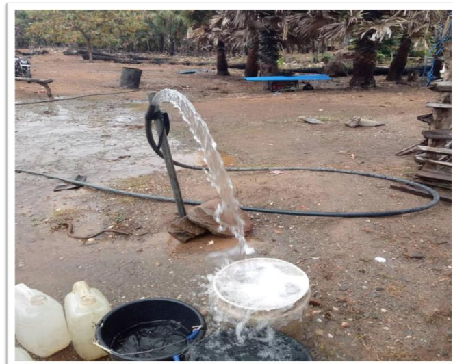
Figure 48: The Water Well Being Built Before the Fence was Erected in Rural Timor-Leste
