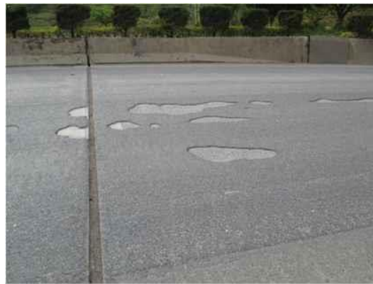
Figure 2.4 Example of delamination
