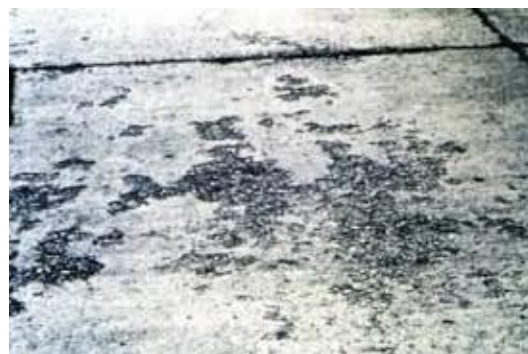
Figure 2.2 Example of scaling and disintegration (adapted from (PCA 2002)).
