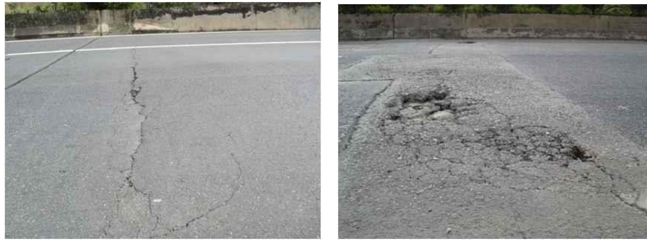
(a) Linear cracking on deck
