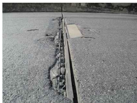
(f) malfunction of expansion joint
