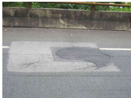
(e) Defects on the pavement
