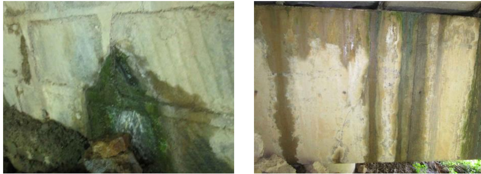
Figure 2.6 Leaching and deposits on concrete
