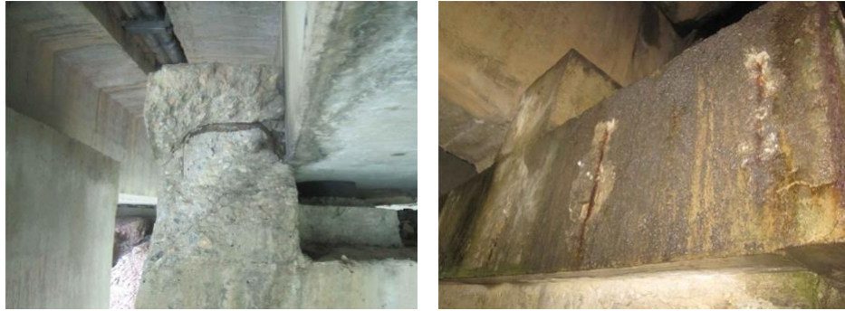
Figure 2.5 Exposed reinforcement with corrosion
