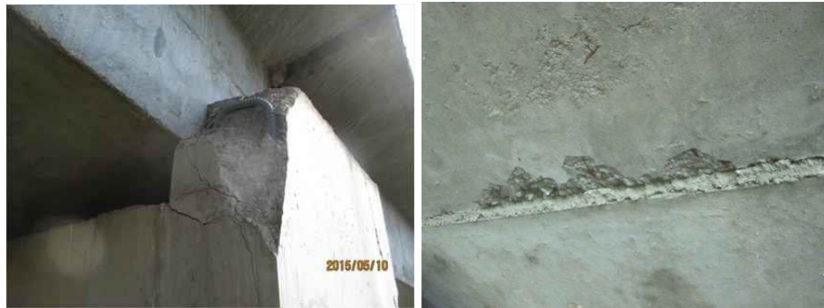
(a) Spalling with exposed reinforcement
