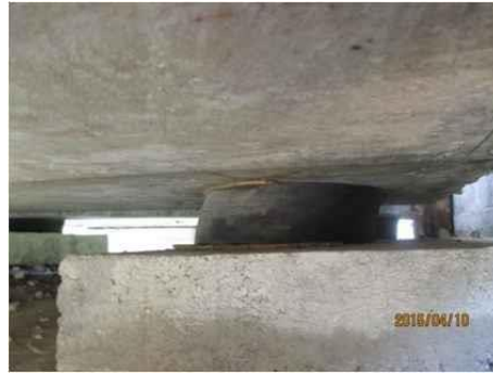
(a) Deformation of bearings
