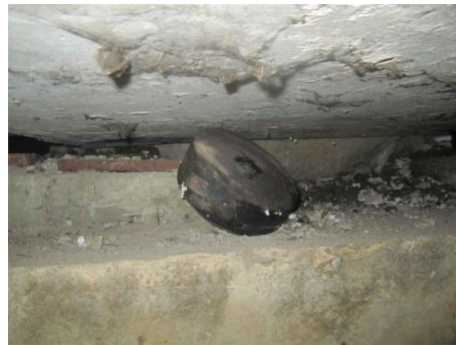
(c) Missing bearings
