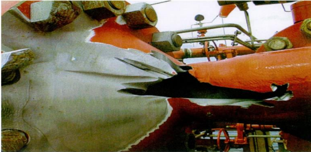
Figure 2-4: An example of loss of containment due to sand erosion [2]
