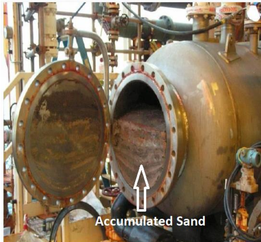
Figure 2-1: An example of accumulation of sand in downstream facility inside a vessel [12]
