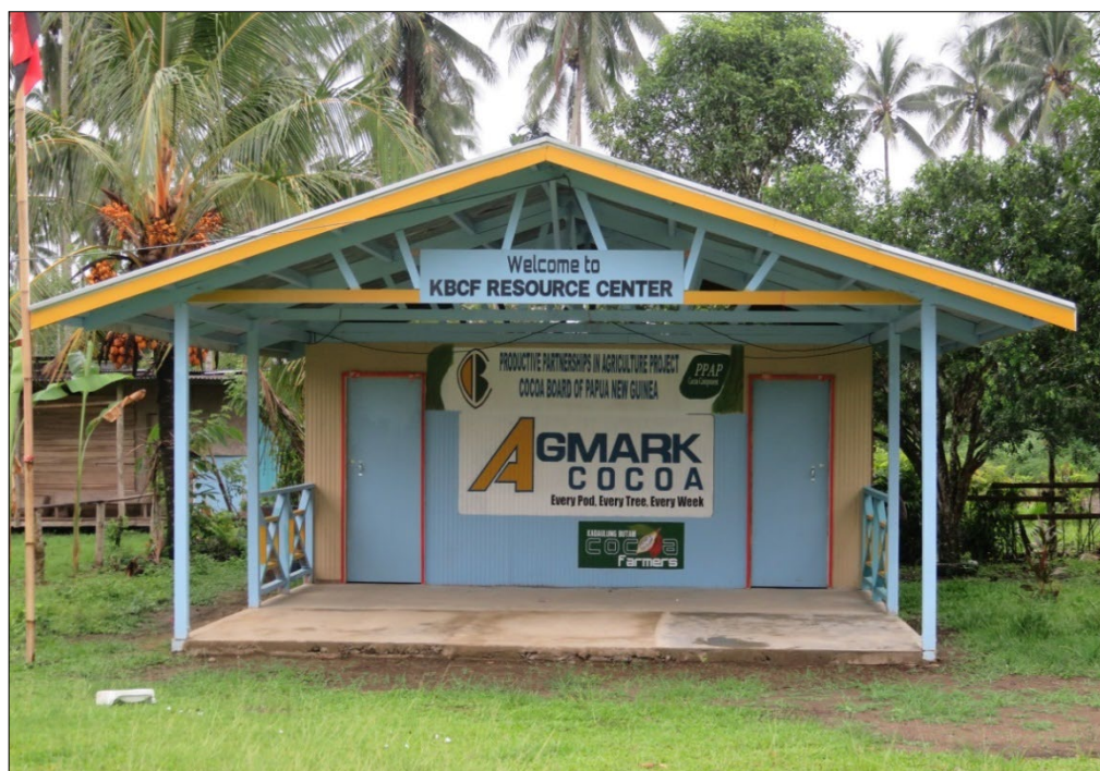
Plate 5.7: A farmer group resource centre under construction by NGIP-Agmark through the PPAP cocoa project
